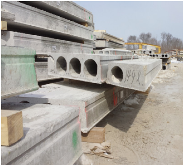
Uneven stacking; dunnage not aligned
