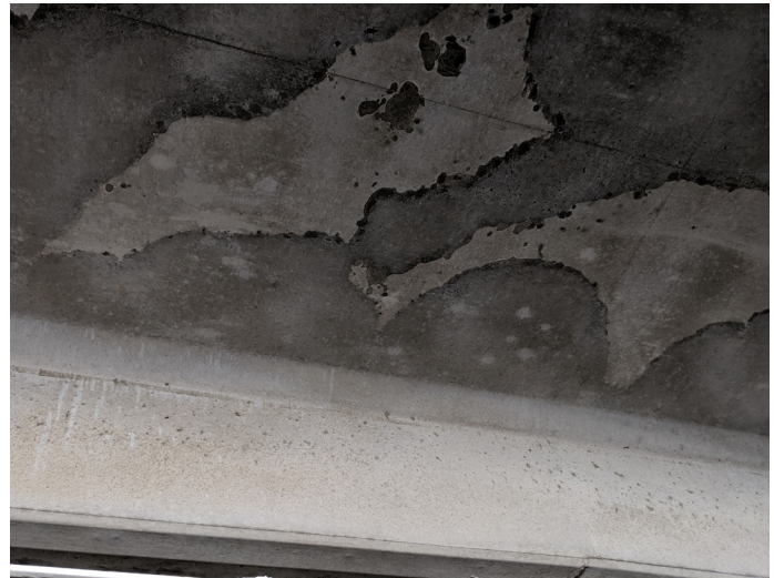
Double tee exhibiting significant pour lines.
