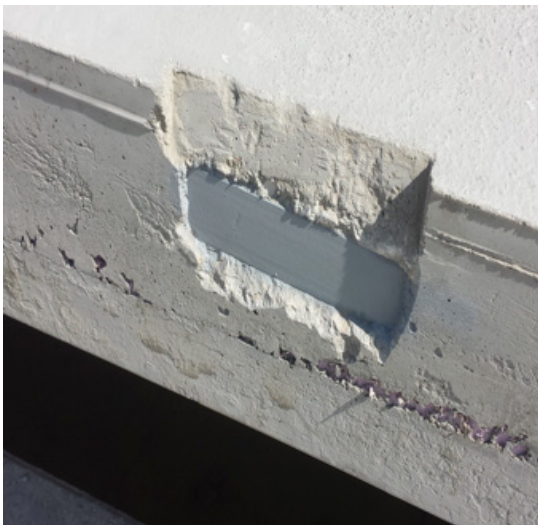
Embed not flush with concrete surface
