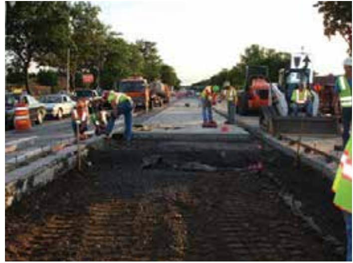
Figure 8-27. An example of undercutting 1 foot prior to replacement with geo-fabric, new subbase material and JPrCP panels.
