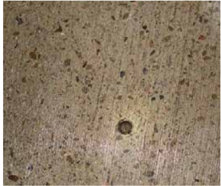
Figure 12-11. This bedding grout port was not properly filled during initial panel installation.
