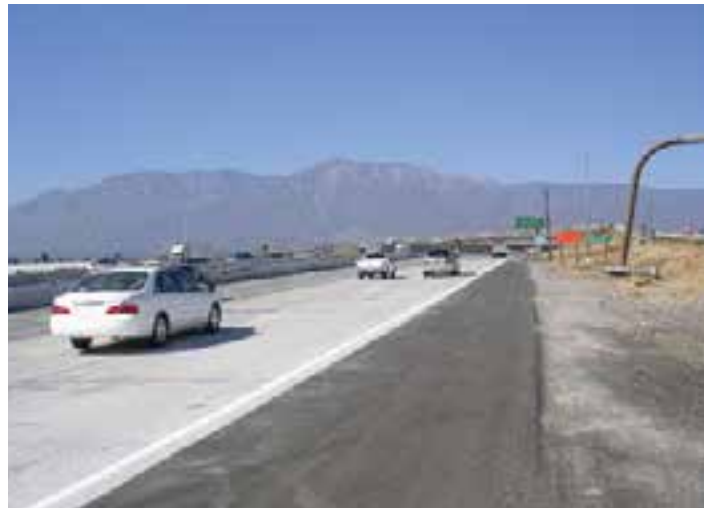
Figure 3-8. Tangent lane replacement of a portion of Interstate 15 near Ontario, Calif., using JPrCP.
