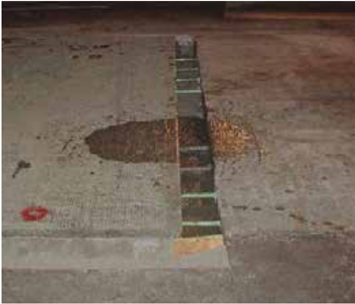
Figure 12-5. This excessively wide transverse joint resulted from cutting the existing pavement (on the right of the joint) at the incorrect location. The dark material at the center of the joint is backfill grout that spilled onto the adjacent slabs during installation.
