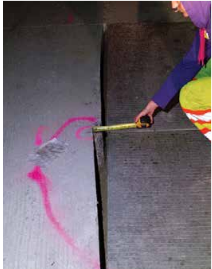
Figure 8-13. Example of an inaccurately sawed longitudinal joint.
