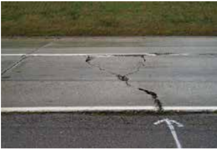
Figure 2-8. Deteriorating transverse crack on concrete pavement.
