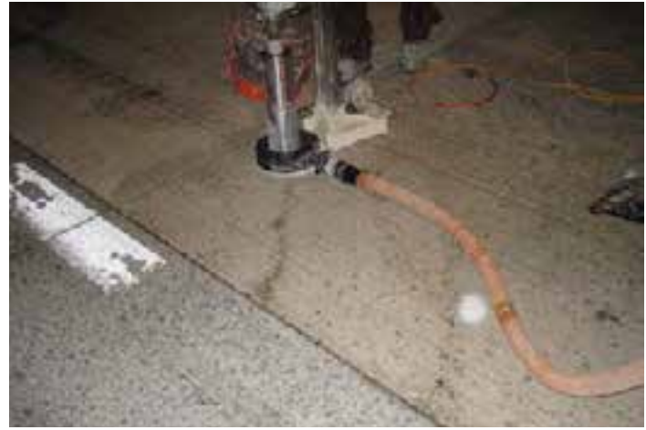
Figure 11-7. This diagonal crack – visible because it is wet – emanated from a bottom slot directly under the core drill. The crack was likely caused by inadequate corner support resulting from improper grading and/or installation of bedding grout.
