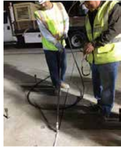
Figure 11-36. Silicone sealant being applied through a nozzle attached to a pressurized drum.
