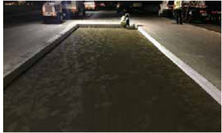
Figure 11-29. 1/2-inch-thick white isolation foam attached to the longitudinal edge of the existing pavement.
