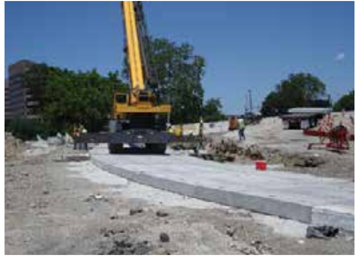
Figure 3-10. “Tight-radius” single-lane ramp in Chicago, Ill., that was replaced during a single weekend closure.
