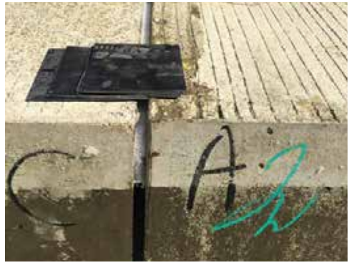
Figure 10-9. Two shims left behind indicate an actual vertical differential of 1/8 inch between the two panels.
