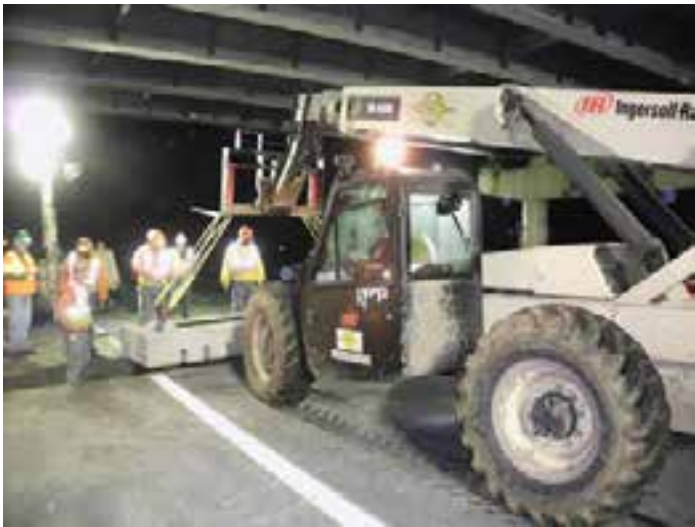
Figure 2-6. Example use of a fork truck to install PCP panels beneath an overpass.
