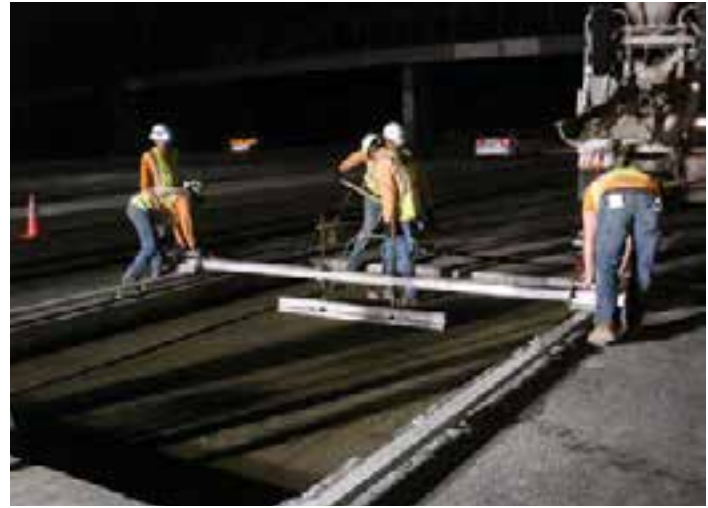
Figure 9-2. Workers use rails set to specific elevations to provide an accurate grade reference irrespective of the undulating existing pavement underneath.
