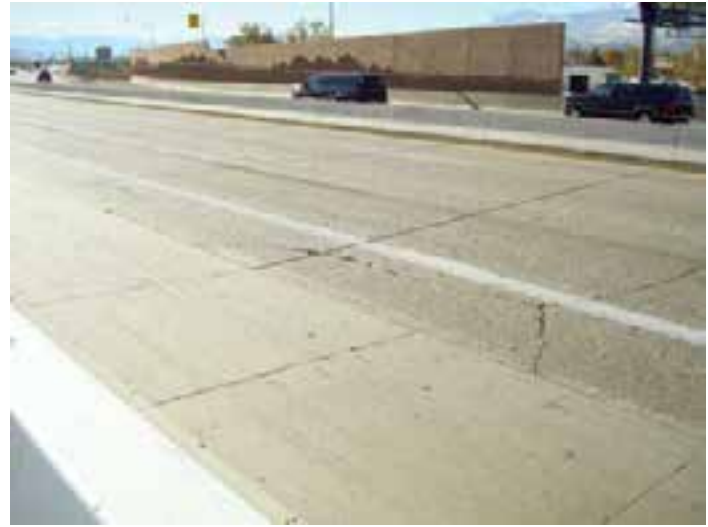
Figure 2-13. Precast panels placed next to cracked panels on Interstate 395 near Reno, Nev.
