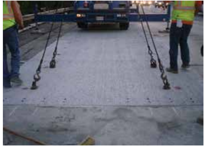
Figure 9-53. All the panels in the lane replacement repair area shown here were placed to leading end marks so the last panel being set precisely fits the space left by the previously placed transverse saw cut.
