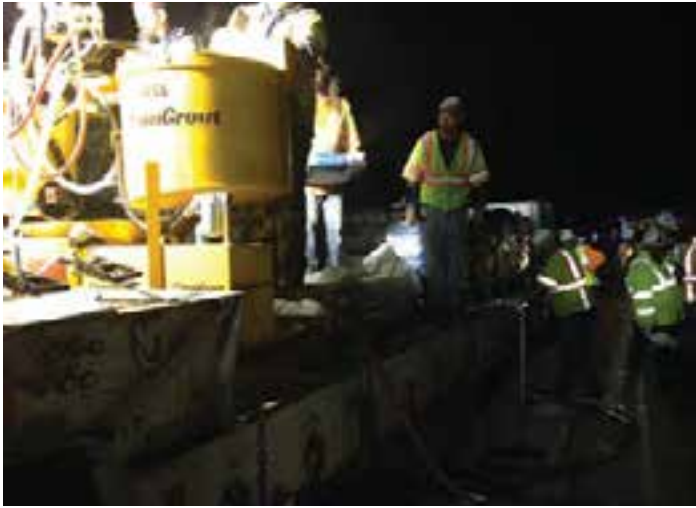
Figure 9-19. A dual-drum, high-capacity mixer/pump mounted on a service trailer with an adequate supply of grout and water and a safe working space.
