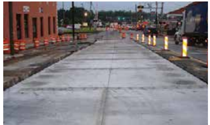
Figure 11-25. Severe cross-slope and vertical profile grade changes at the far end of new panels.
