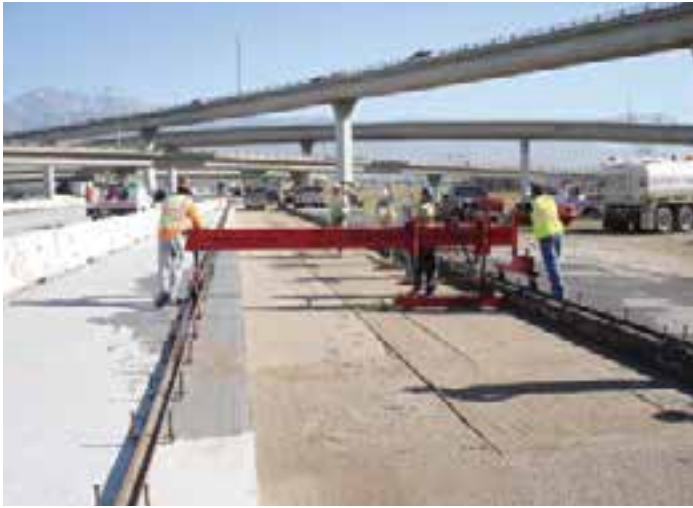
Figure 9-3. A larger, hand-operated grader controlled by pre-set grade rails set to specific elevations.
