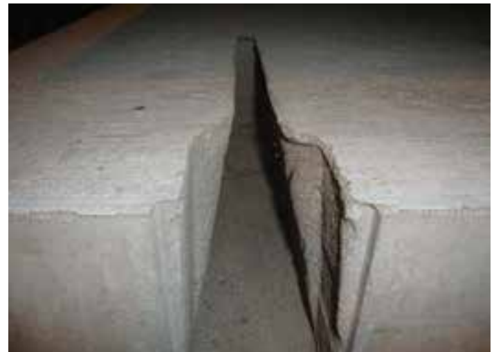
Figure 9-33. Slot openings in the Illinois Tollway system are dovetail in shape (narrower at the top than at the bottom).
