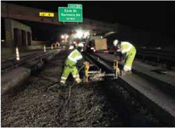
Figure 9-41. A single-bit air drill used for drilling tie bar holes at correct locations.
