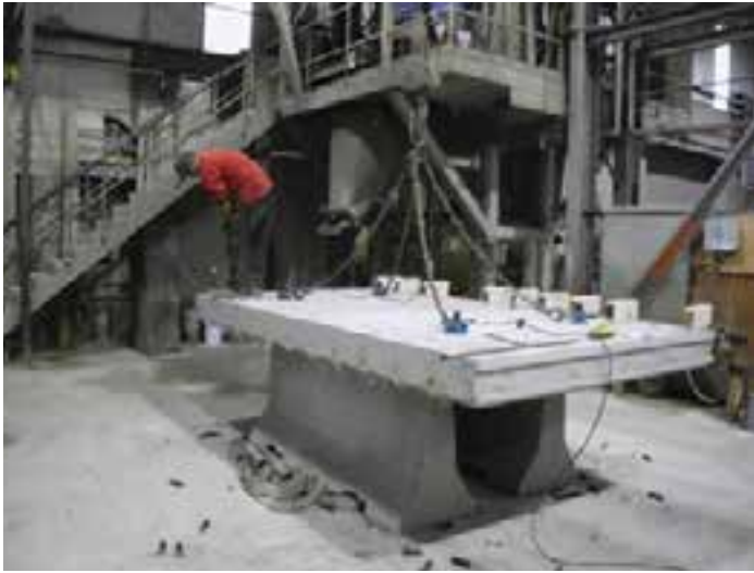
Figure 7-26. Panel placed on waist-high stands to facilitate stripping of slot formers, post-pour checking and panel detailing.
