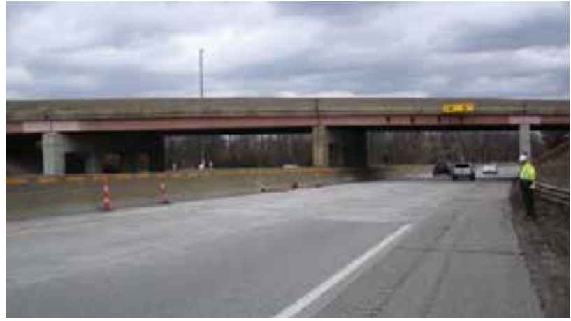
Figure 3-27. Completed repairs beneath an overpass on eastbound Interstate 94 (Business Loop) near Kalamazoo, Mich.
