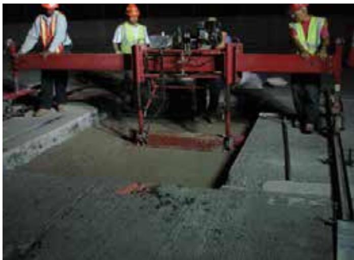
Figure 11-1. The relatively thin spall in the existing pavement seen along the longitudinal joint in the lower-right corner was caused by improper removal techniques.
