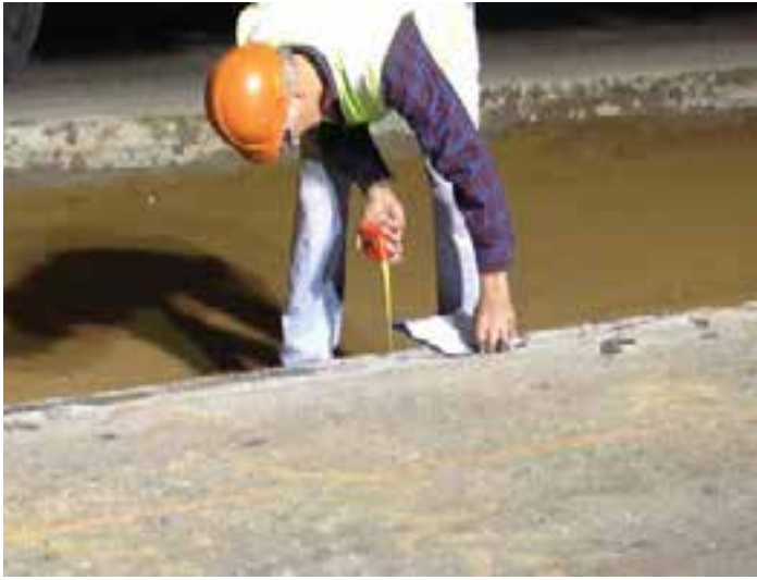
Figure 10-10. A DOT inspector checks the finished elevation and grading of the subbase.
