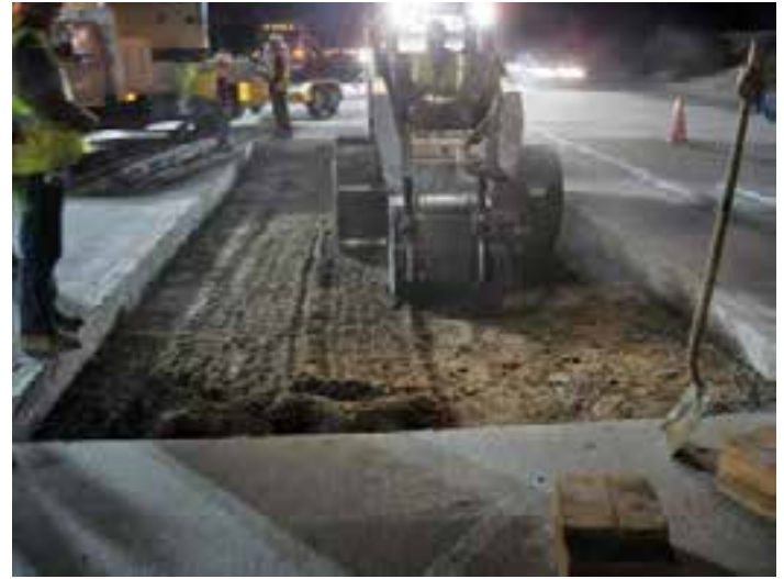
Figure 2-15. Removal of cement-treated base using a skid-steer-mounted milling machine on Interstate 210 in Tarzana, Calif.
