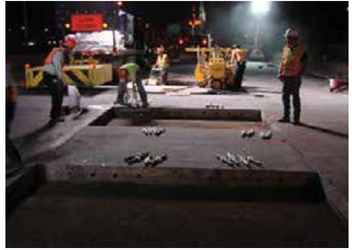
Figure 3-5. Construction of precast panel repairs for joints and mid-slab cracks in 40-foot-long panels.
