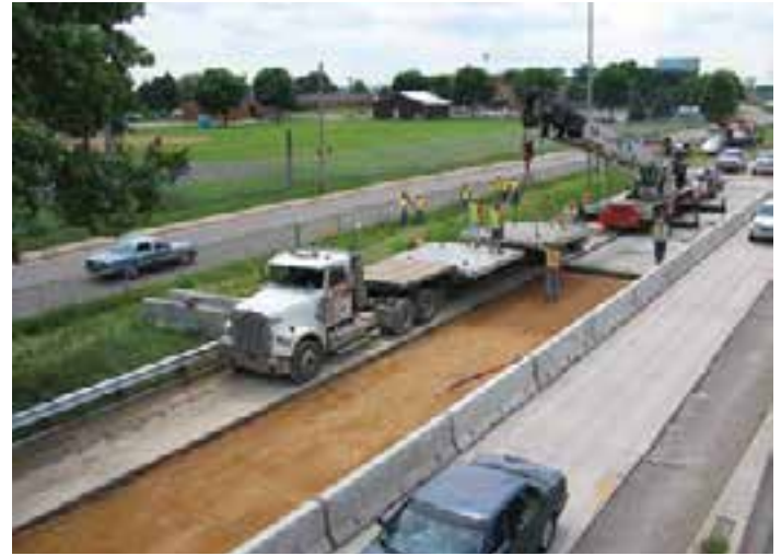
Figure 9-46. A 65-ton capacity hydraulic crane picking panels from a truck positioned in front of, rather than alongside, the crane.
