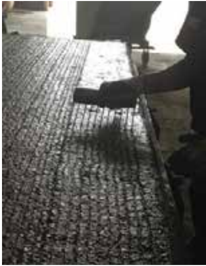
Figure 7-24. Use of a narrow, custom-width rake to texture a narrow strip at the edge of a panel.
