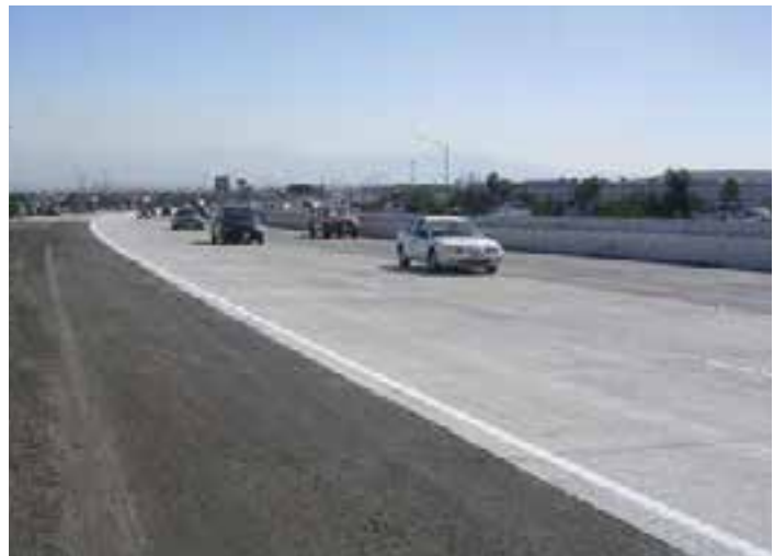
Figure 3-9. Lane replacement of a curved portion of Interstate 15 near Ontario, Calif., using JPrCP.
