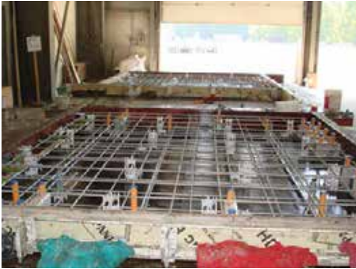
Figure 1-8. Two layers of reinforcing steel in each direction in a JPrCP fabrication.
