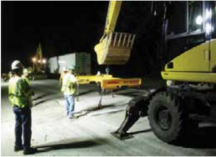
Figure 9-47. The outrigger of this rubber-tired excavator is located outside of the PCP panel area.
