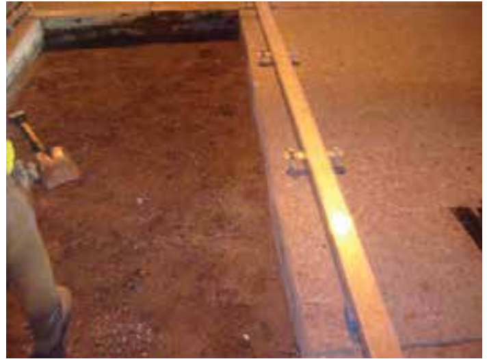
Figure 8-18. An undulating vertical saw cut made with a blade that was likely too flexible for the pavement.
