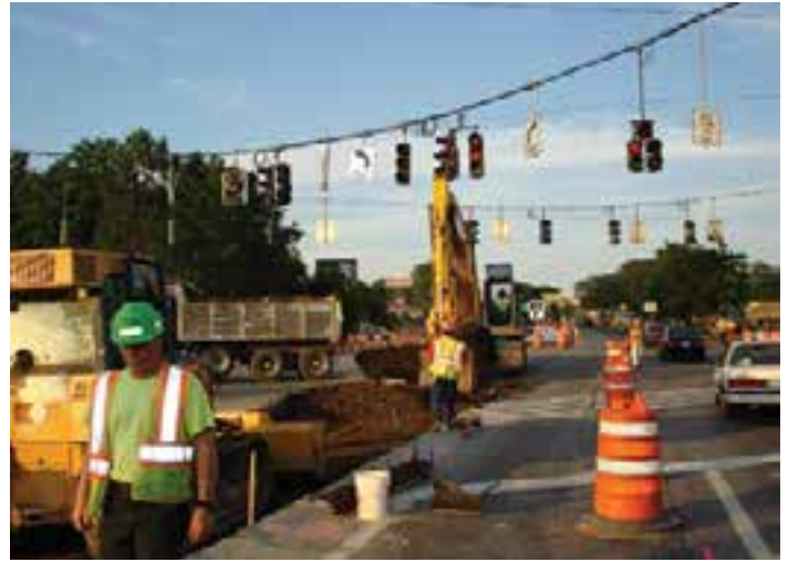
Figure 3-15. Street view of pavement replacement operations at the intersection of Route 7 and Nott Street in Rotterdam, N.Y.
