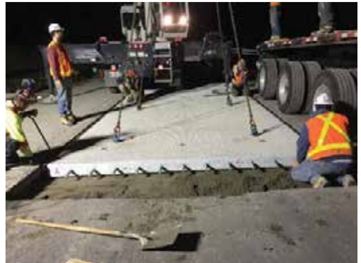
Figure 13-17. A precast panel being placed in the grade-supported section of the project.
