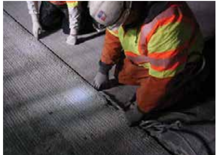
Figure 11-32. Small-diameter backer rod being braided together to fill a variable-width longitudinal joint prior to sealing.
