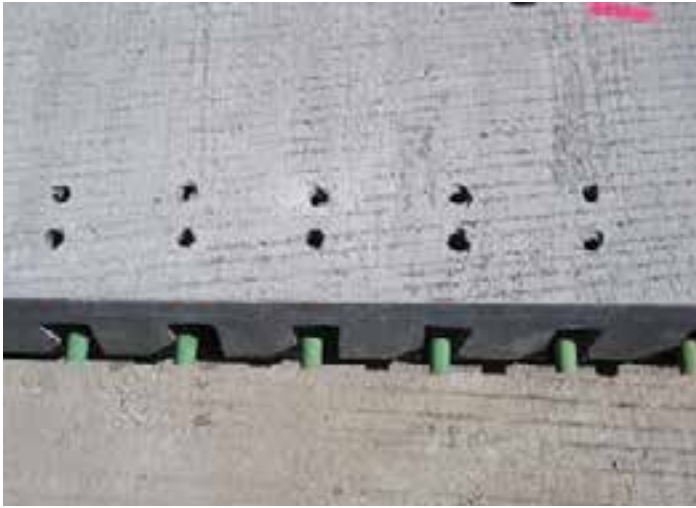
Figure 9-23. A Super-Slab panel being lowered over the dowels of a previously placed panel.
