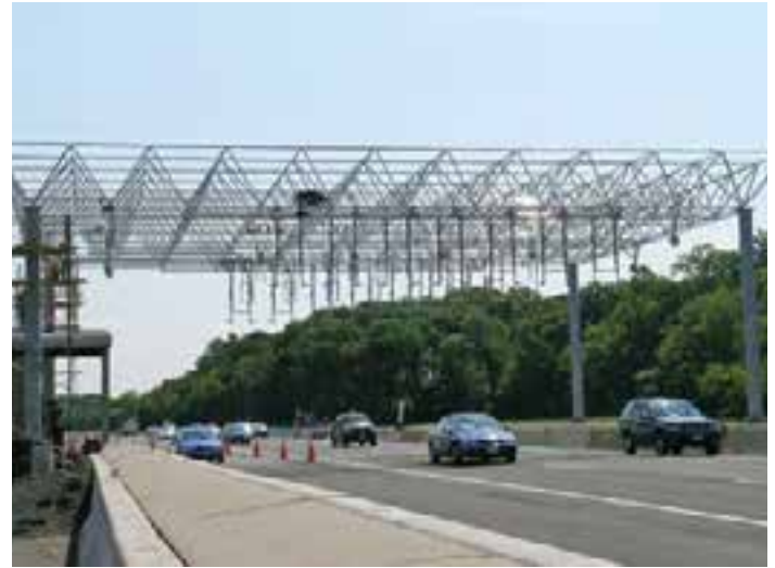
Figure 13-24. Overhead open-road-tolling equipment integrated with treadles embedded in precast panels below at New York Thruway Spring Valley toll plaza.
