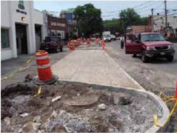
Figure 13-20. Non-planar, specially shaped precast panels were manufactured to meet the adjacent granite curb and pronounced surface contours while providing continuous commercial access.
