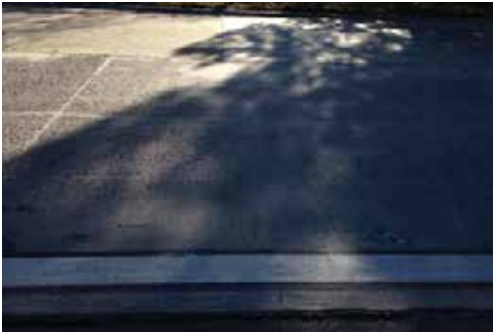
Figure 11-6. A transverse crack in the foreground lane lines up approximately with a joint at a cast-in-place concrete patch in the adjacent lane.
