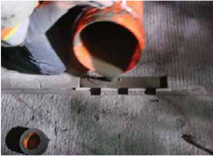
Figure 11-3. Two layers of foam (with black tape adhered to the near panel) were used along this transverse joint to retain the joint reservoir for the joint sealing material while repair material was installed.
