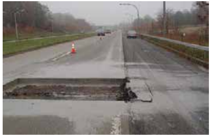
Figure 8-14. Failure to cut the asphalt shoulder prior to pavement removal resulted in serious shoulder damage on this project.
