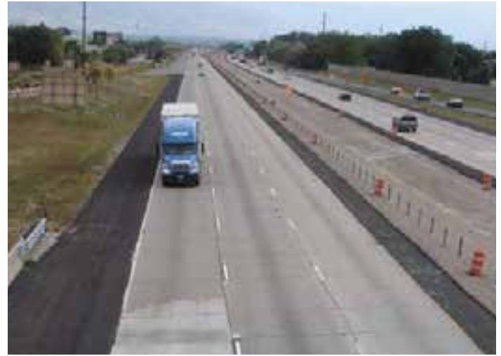
Figure 11-24. The existing pavement in the lower left corner of this photo was ground on both the approach and leave ends of a panel because the precast panel was placed too low.
