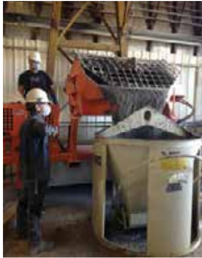
Figure 13-21. Mixed polymer concrete being discharged from a mixer into a concrete bucket.
