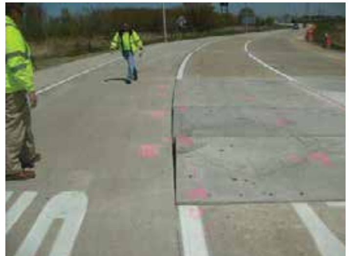
Figure 8-11. Example of a “saw-tooth” longitudinal joint created because the end cut, seen in the foreground, was not laid out and cut radially to the horizontal curve.
