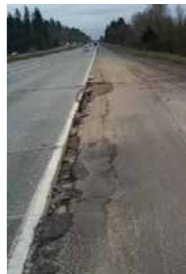
Figure 2-11: Joint and crack faulting with severe pumping, indicating drainage and erosion problems.
