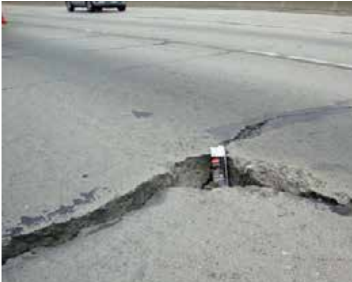
Figure 1-1. Photo of deteriorated concrete pavement.
