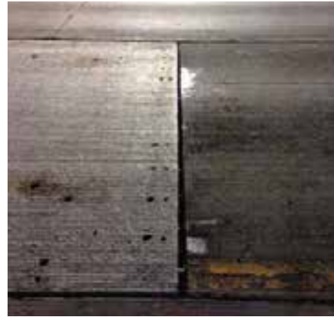
Figure 11-12. The transverse joint seen here varies in width from about 1/2 inch on the far end to approximately 2 inches on the near end because of incorrect saw cutting of the existing pavement.
