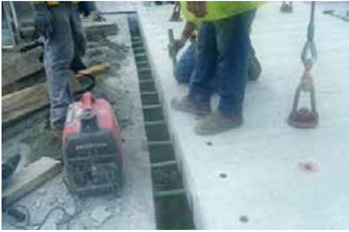
Figure 11-11. The over-width transverse joint in this photo resulted from incorrect saw cut layout in the existing pavement on the left. The error was not discovered until the precast panel on the right was placed.
