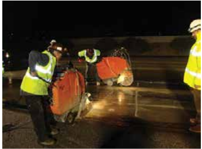
Figure 13-14. A transverse saw cut being made at the terminus of a single night’s installation. An additional saw making the longitudinal cut is seen in the background.
