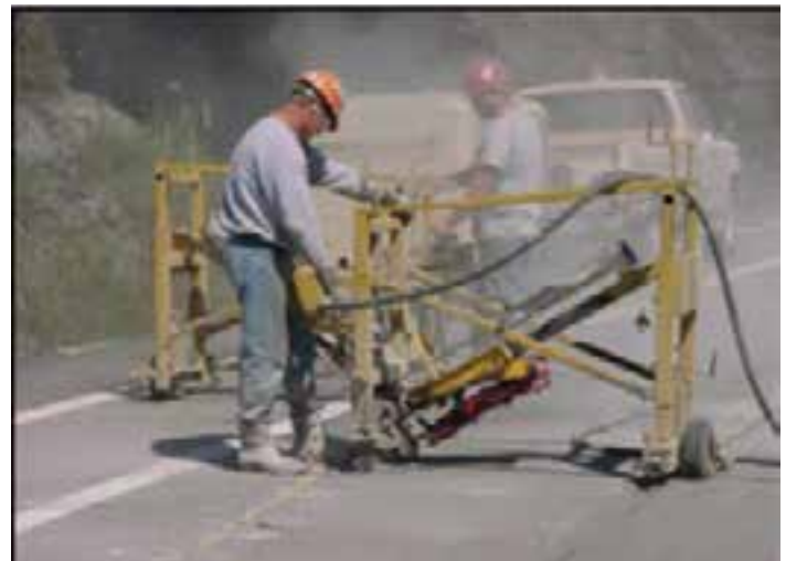
Figure 9-40. A worker uses a pneumatic drill to create cross-stitch holes across a longitudinal slab crack.
