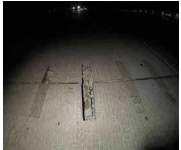
Figure 12-4. Bond failure between the grout encasing the dowel and the vertical sides of the slot.
