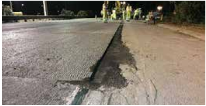
Figure 11-37. This new asphalt – placed directly against new precast panels – was barely wide enough to allow proper and uniform compaction.
