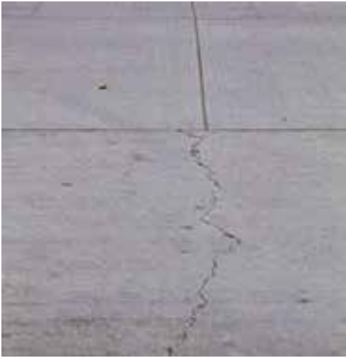
Figure 4-1. Transverse sympathy cracking due to mismatched transverse joints.
