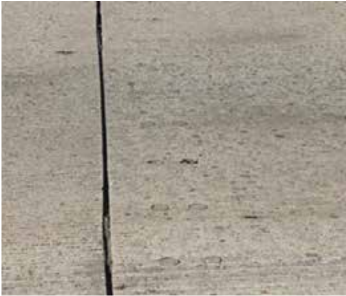
Figure 12-10. Grout in some dowel grout ports may have de-bonded here, potentially allowing water to penetrate to the dowel bar level.
