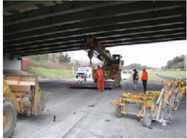
Figure 2-5. Example use of an excavator placing PCP panels beneath an overpass. Traffic is maintained on the lane to the right of the excavator.
