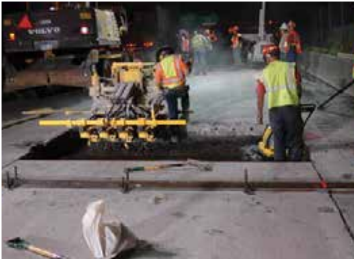
Figure 9-37. Holes for new dowels in this photo are evenly spaced at a uniform distance from the top of the existing pavement, ready for insertion and anchoring of dowels.
