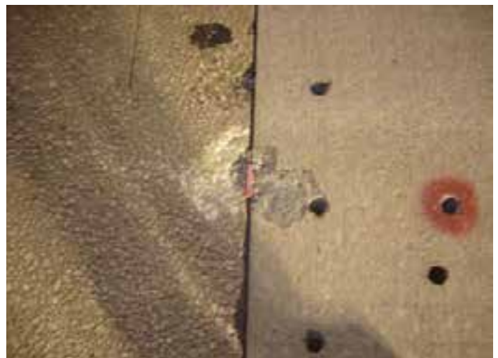
Figure 11-2. Transverse joint spalls in both the existing pavement and the new precast panel in this photo resulted from the red shim pad – placed to keep adjacent panels from hitting each other – being placed too close to the surface.
