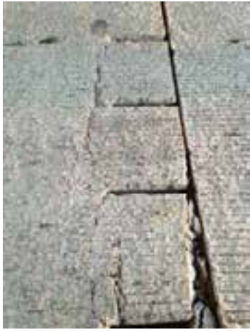
Figure 11-15. This photo shows a cast-slide panel that shattered around the dowels before the slots were grouted.
