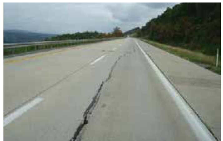
Figure 2-10: Longitudinal crack (possibly due to foundation support issues).
