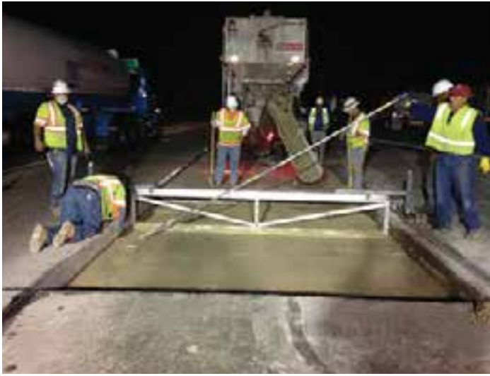
Figure 10-14. Two concrete finishers working behind four workers screeding newly placed lean concrete subbase.
