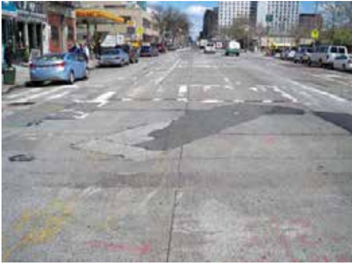
Figure 13-10. An example of city street pavement with many utility cuts (First Avenue, New York City).
