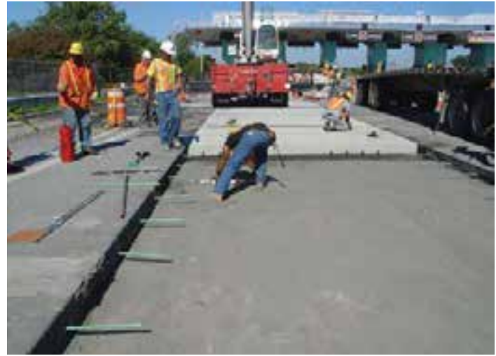
Figure 9-48. Both sets of outriggers on this hydraulic crane are positioned on existing pavement.
