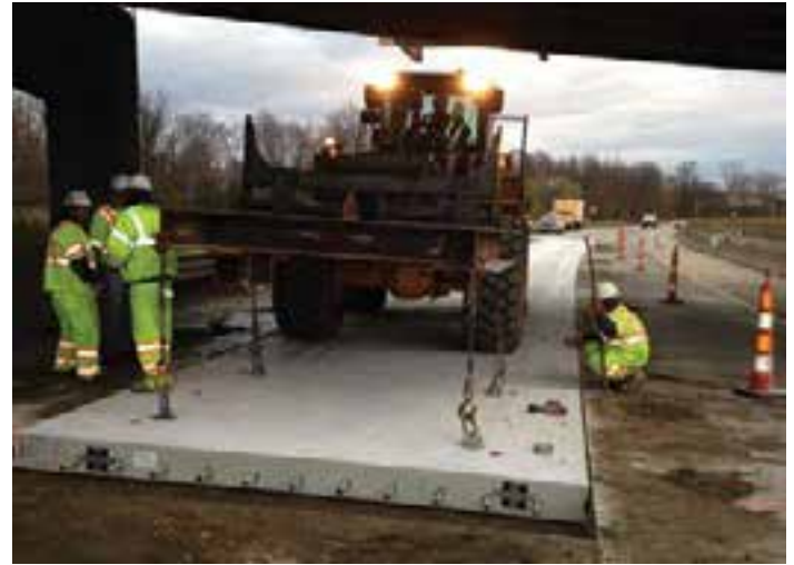
Figure 9-51. A large loader carrying and placing a PCP panel under an interstate overpass.
