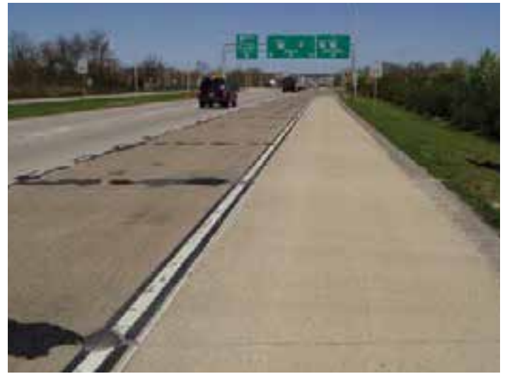
Figure 2-9. Joint failure on concrete pavement.
