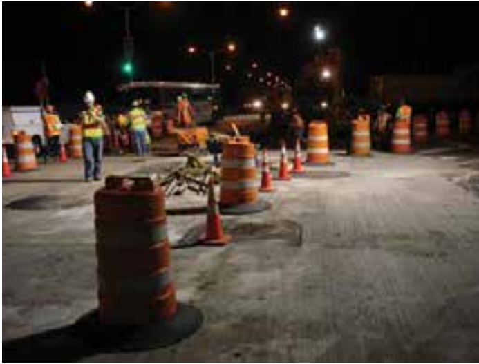
Figure 2-18. Numerous utility blockouts in precast panels temporarily filled with asphalt to maintain traffic.
