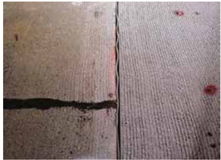
Figure 11-30. The isolation foam in this longitudinal joint does not completely fill the joint.
