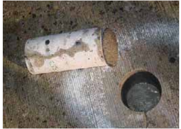
Figure 11-10. The crack in this core measured .06 inches wide at the top of the core and stopped at the bottom layer of reinforcing.
