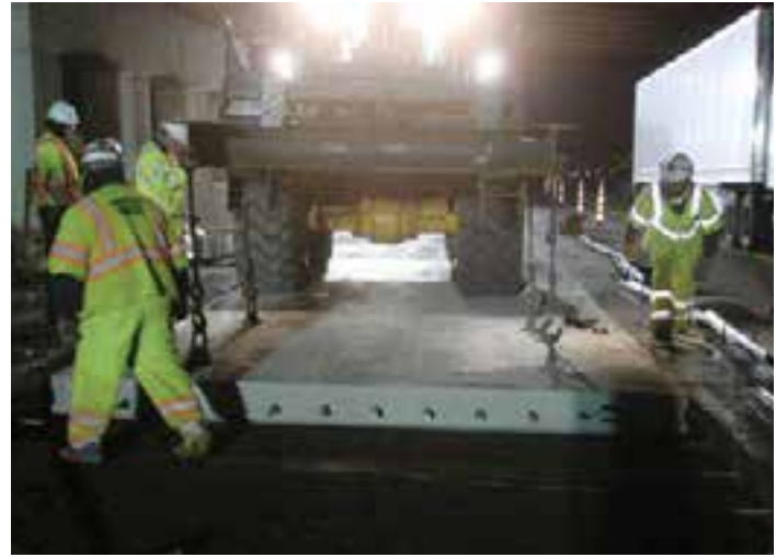
Figure 9-42. Installation of a bottom-slot precast panel over tie bars drilled in vertical faces of adjacent existing pavement.
