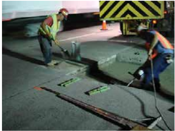
Figure 8-3. The narrow buffer zone in this two-lane working area required workers to exercise extreme caution.
