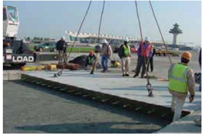
Figure 3-32. Installation of precast taxiway panels on precision-graded base at Dulles International Airport.
