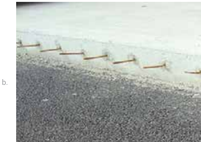
Figure 4-17. Schematic of a tied longitudinal construction joint with optional keyway and photo of tie bars along longitudinal joint. Sources: a. American Concrete Pavement Association; b. Pavement Engineering and Research Associates, LLC
