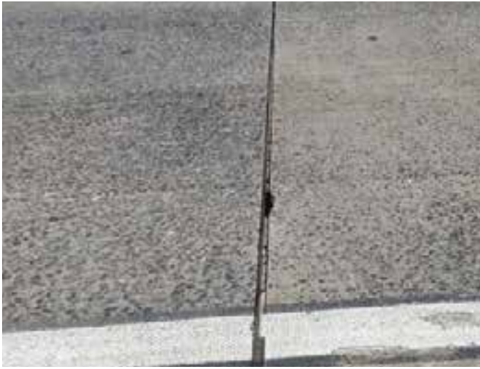
Figure 12-8. Joint-filling grout between the silicone seal on the left and the panel on the right has de-bonded from the panel, creating a maintenance problem in this variable-width joint.
