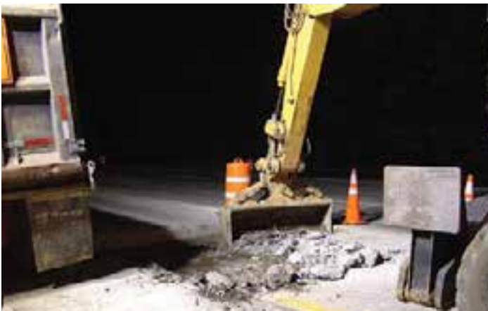
Figure 8-24. The shattered pavement seen here had to be removed with an excavator even though the lift-out method was specified.
