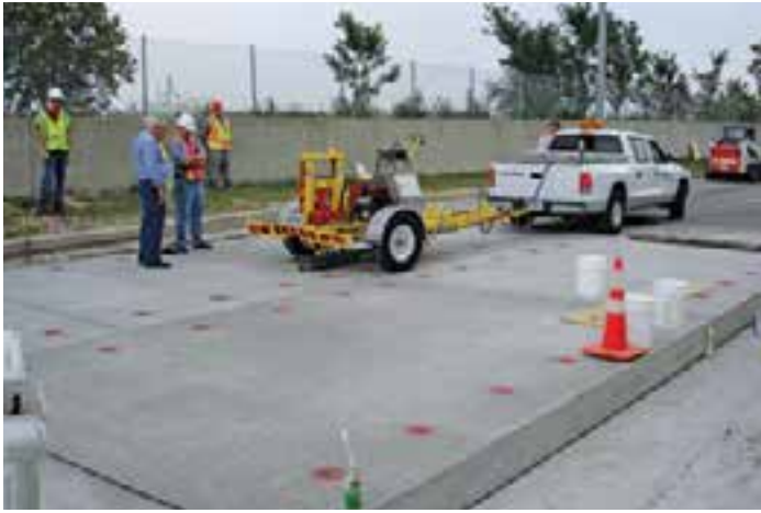
Figure 10-2. Falling weight deflectometer equipment measuring load transfer efficiency at a trial installation in Chicago, Ill.
