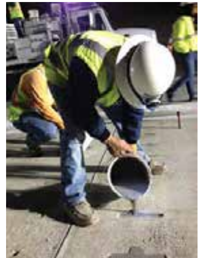
Figure 9-32. Latex grout being poured into the narrow top slot of the Barra Glide system.
