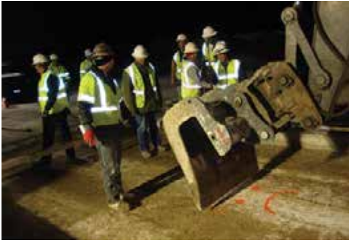
Figure 8-31. Trimming isolated high spots in CTB (red marks) with an excavator bucket.
