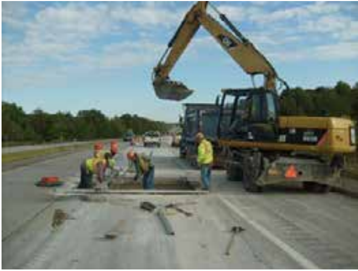
Figure 8-26. The versatile rubber-tire excavator can be used for removal, rough grading and placement of new panels up to 10 feet by 12 feet.
