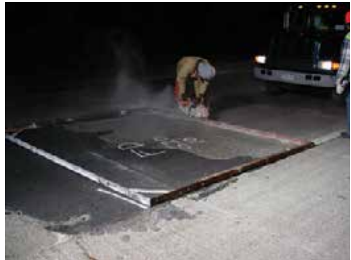
Figure 8-8. An example of a contractor-designed steel template being used to lay out and score saw cut lines for a single panel.
