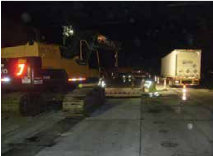
Figure 9-50. A track-mounted excavator placing a PCP panel under an overpass on Interstate 94 in Kalamazoo, Mich.
