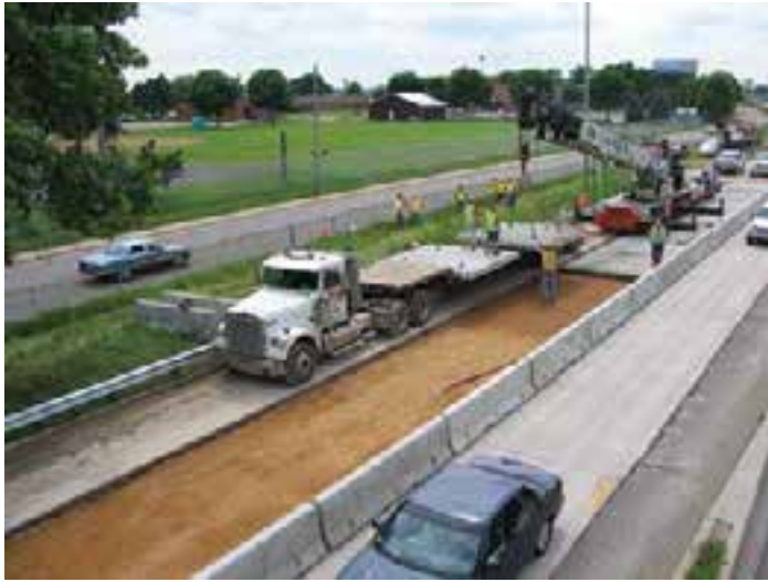
Figure 2-2. Example use of two lanes to perform repairs in a single lane.
