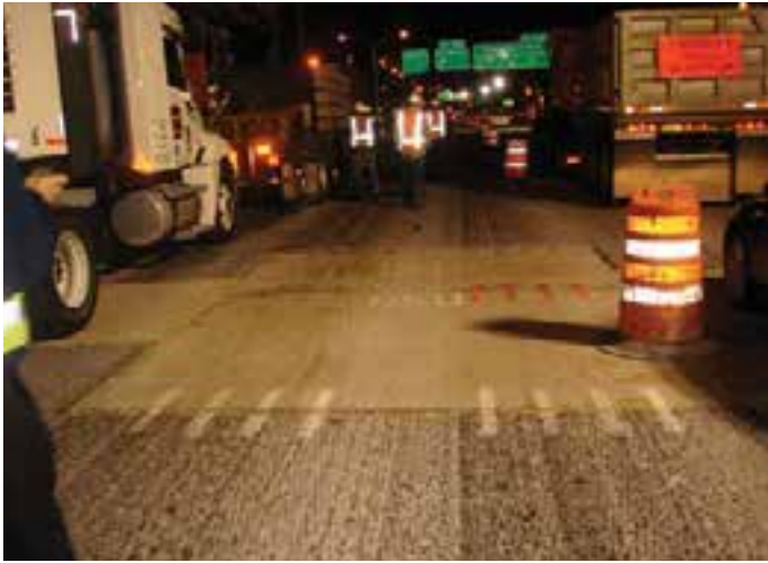
Figure 9-21. Two newly installed panels marked out for field saw cutting at precast-to-precast and precast-to-existing joints.
