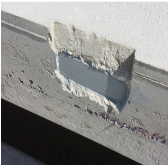
Embed not flush with concrete surface
