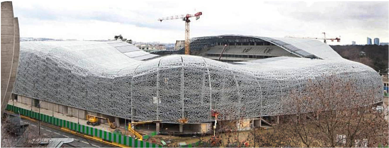
Figure 32 – Mega project: Stade Jean Bouin, a 23,000 square meter UHPC lattice envelope and roof. (Photo: Nanick Guihodo)
