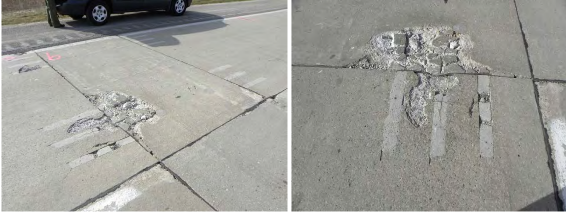
Figure 3.6. Views of a deteriorated panel at the I-675 project (planned for replacement).
