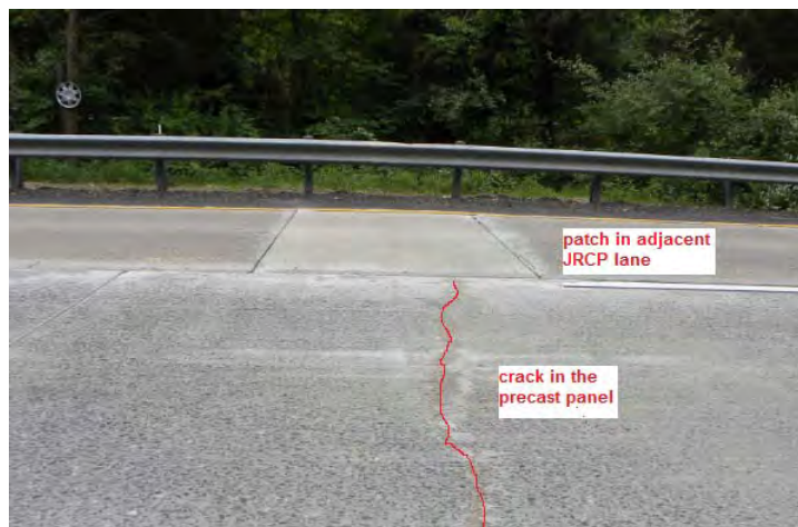
Figure 3.11. Crack in a precast panel associated with a patch in the adjacent lane.
