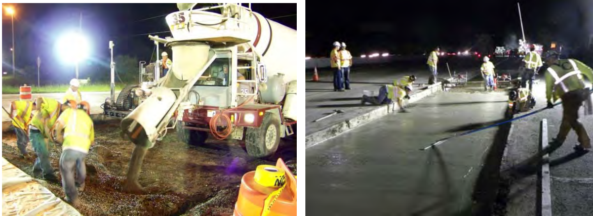
Left: CTPB placement during the Delaware PPCP project Right: LCB placement during the California I-680 PPCP project
