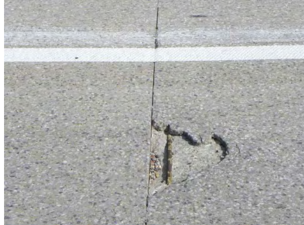
Figure 3.19. Spalling at an intermediate transverse joint.
