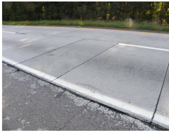
Figure 14.4. View of the I-95 jointed FDRs.
