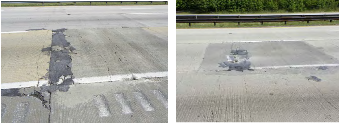
Figure 14.3. Failed FDRs in CRCP.
