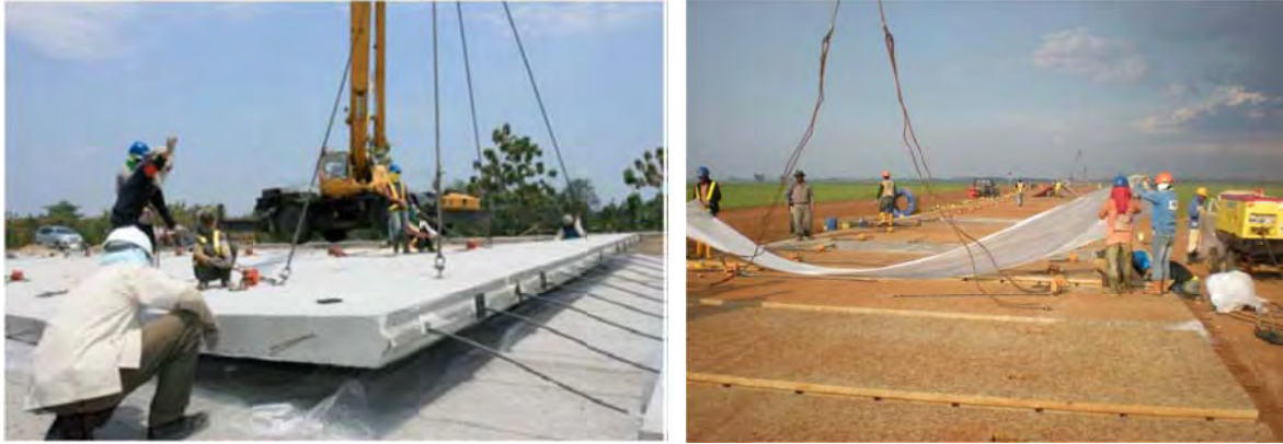
Figure 2.18. Indonesia PPCP installation.
