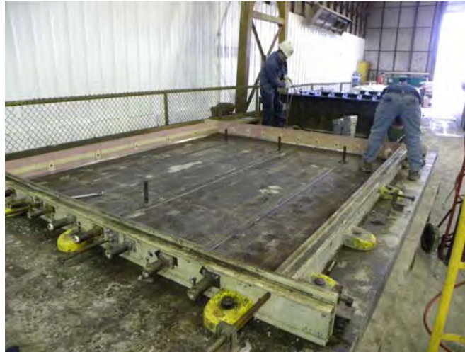
Figure 9.1. Typical formwork used for a continuous jointed PCP system. (Courtesy of FMC)
