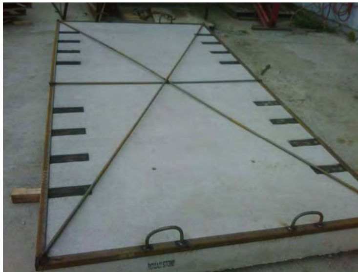
Figure 10.1. Template used for marking the repair area perimeter. (Courtesy of the Roman Stone Construction Company)
