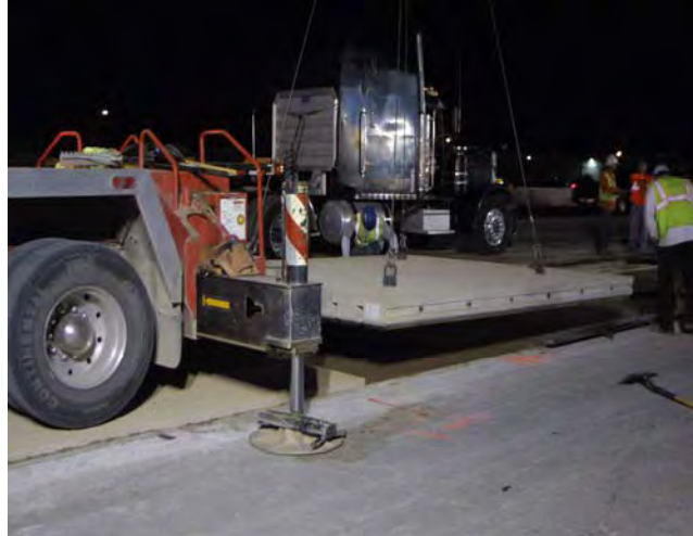
Figure 15.6. Crane stabilization requires 2 to 3 additional feet away from the rehabilitation lane on each side.
