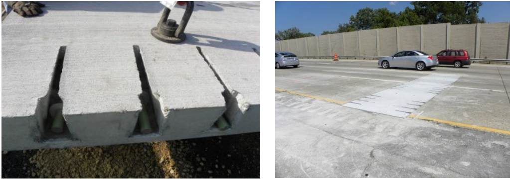
Figure 7. Photos. A repair made using the Illinois Tollway version of surface slot panels.
