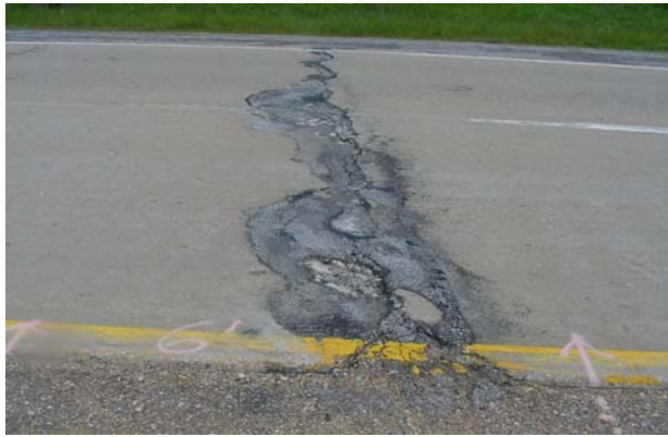
a) Deteriorated joint with cold patch with spalling.
