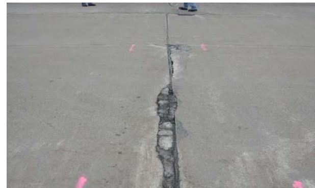
d) Deteriorated joint with spalling.
