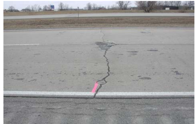
b) Medium-severity transverse crack.
