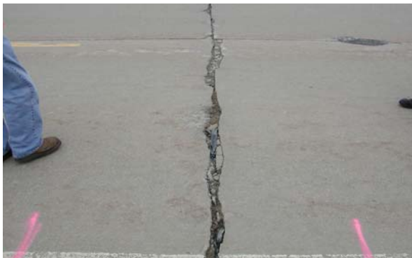
c) High-severity transverse crack.
