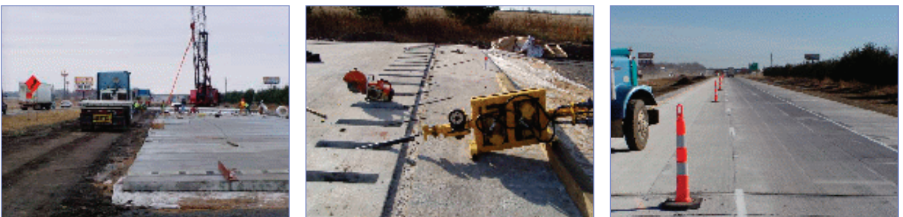
Figure 7. Installation of the precast panels at the Missouri project (left, staging of trucks and installation crane; center, final post-tensioning; right, completed project).
