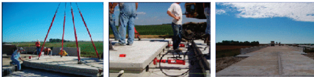
Figure 8. Installation of the PPCP bridge approach on SR 60 (left and center, installation of precast bridge approach slab; right, completed approach slab).
