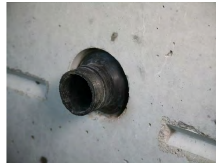
Pipe to Tank Connections
