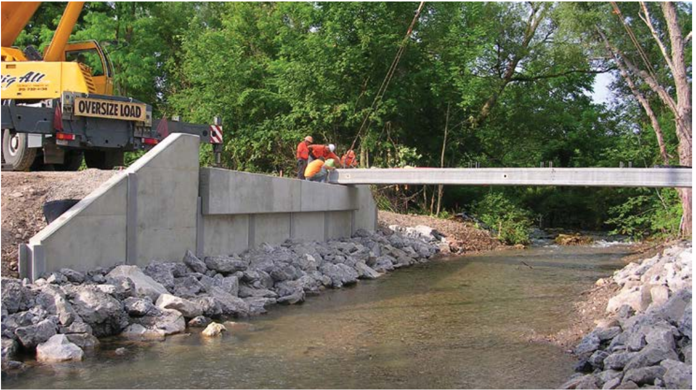
Prestressed beams are set on the south abutment above the precast abutment system.
