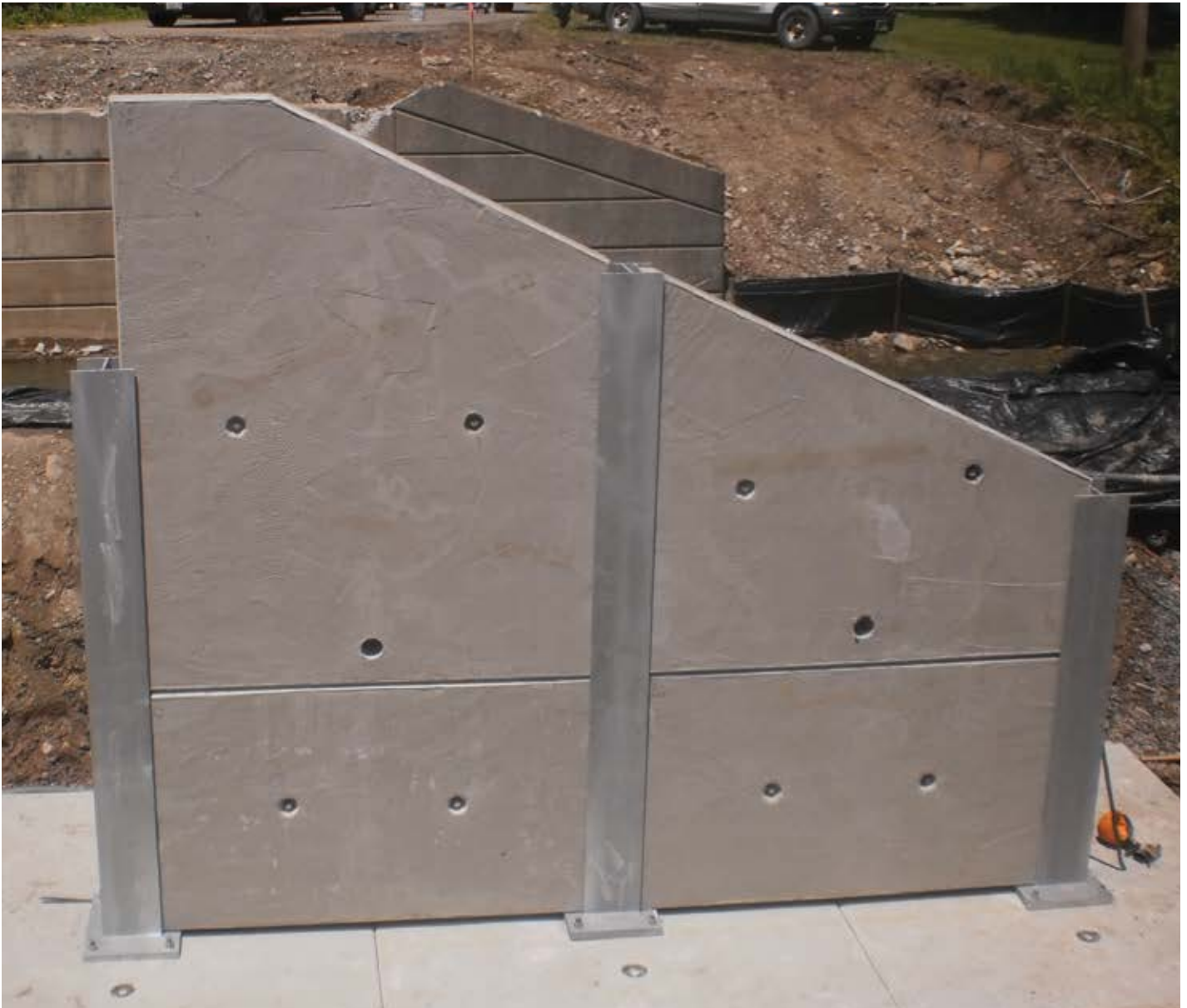
The adjacent wing wall abutment panels are in place for the South Creek Road Bridge.
