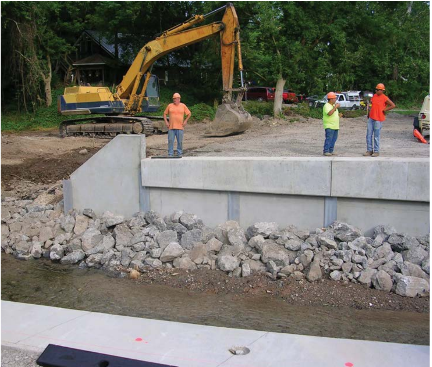
A crew member looks over a finished half of the north abutment of the South Creek Road over Clockville Creek bridge replacement in Lincoln, N.Y.
