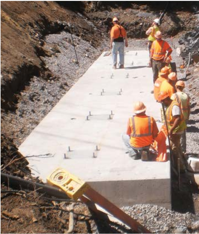
Workers install six footing sections to begin work on the precast abutment system.
