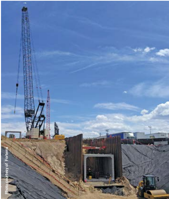
The Globeville Landing Outfall will protect homeowners and property from catastrophic flood damage.
