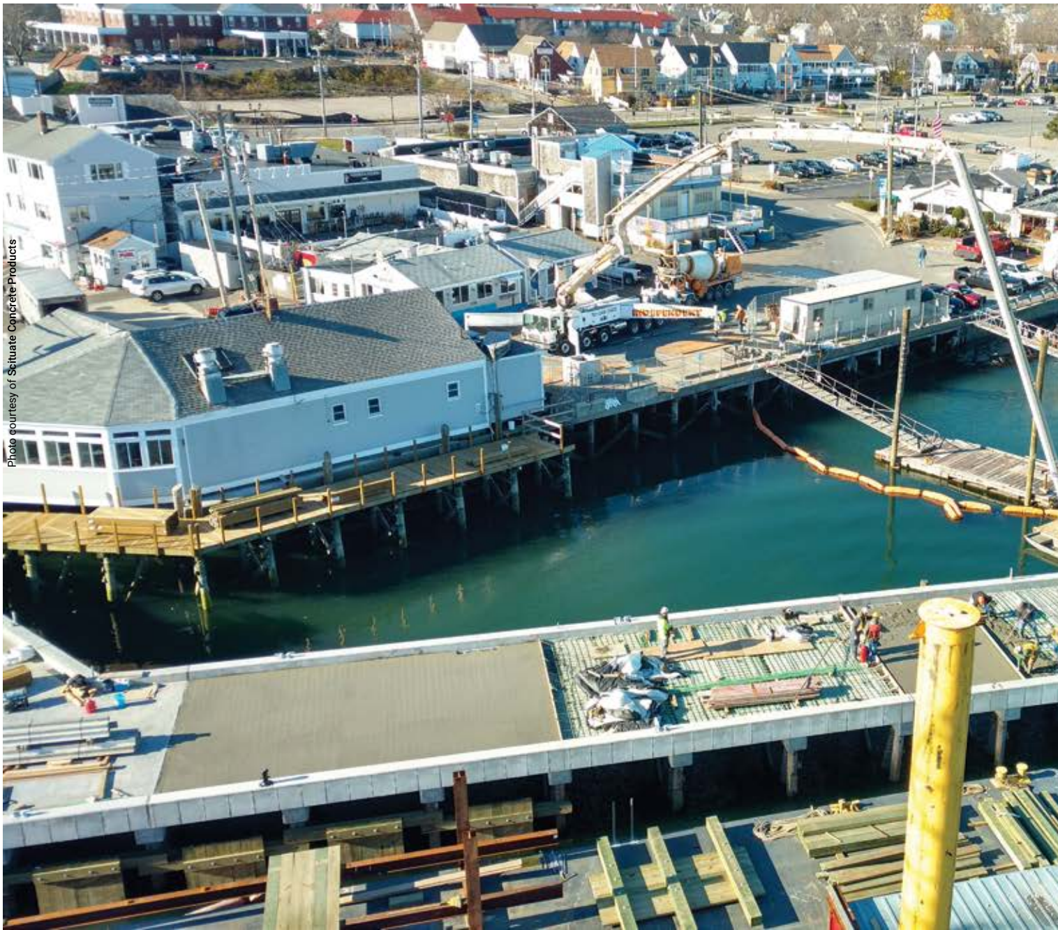
The precast concrete substructure, which includes the massive pier casts, supports the wharf's decking.
