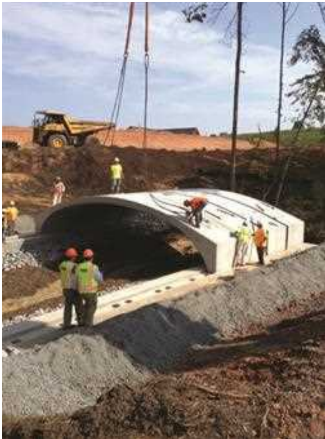
Nearly every underground item at the Tryon International Equestrian Center in Mill Spring, N.C., was constructed and installed by Tindall.
