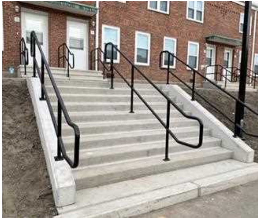
Max Pryor helped install the steps outside Carroll Hall at Central Connecticut State University, from where both he and his sister, Lexi, graduated
