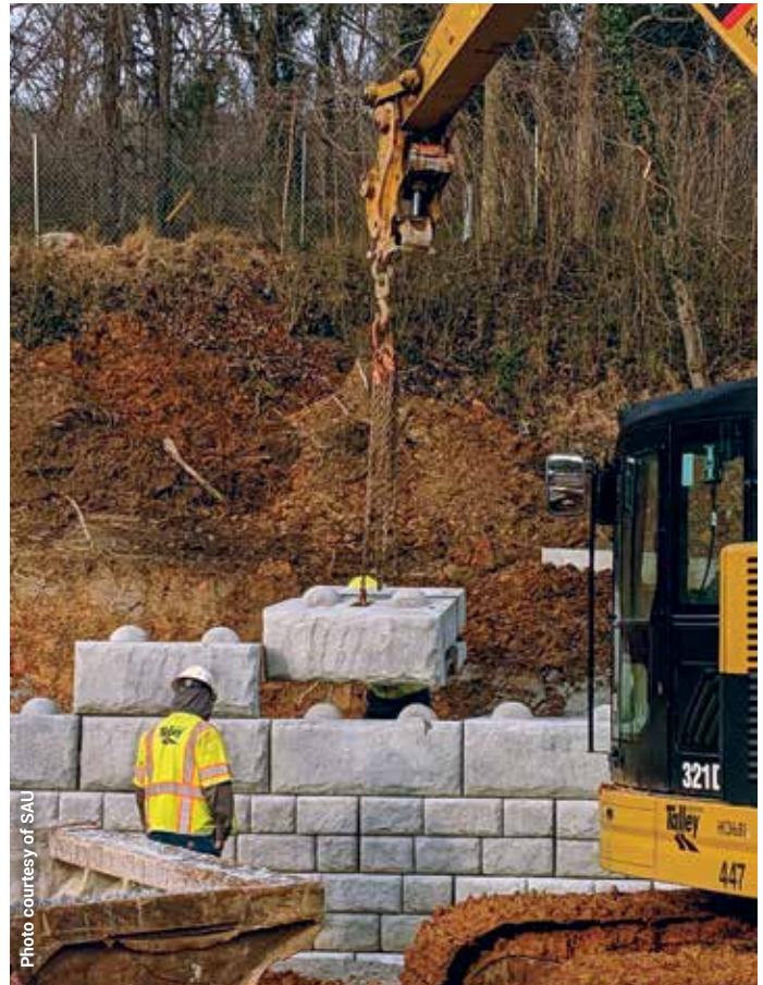
Two walls totaling more than 550 feet long were manufactured for the project.
