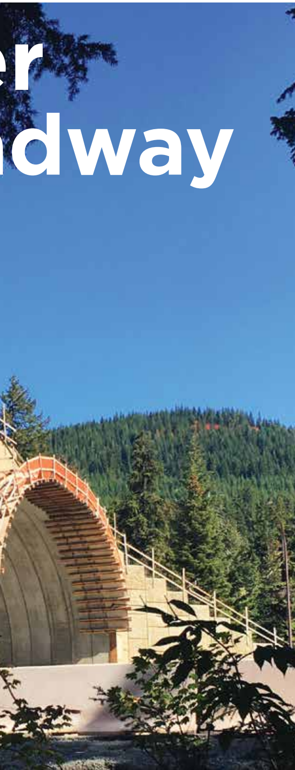
A precast concrete arch system and MSE walls create a safe passage for wildlife in Washington state.
