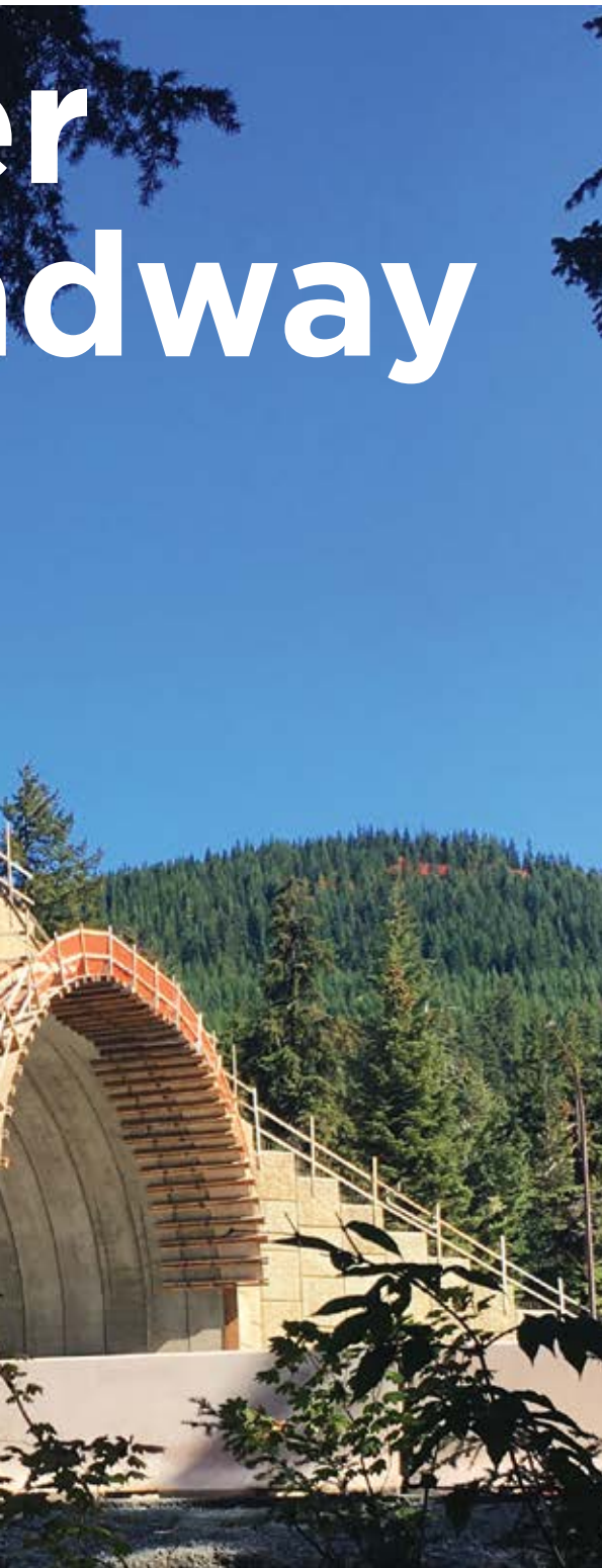
A precast concrete arch system and MSE walls create a safe passage for wildlife in Washington state.
