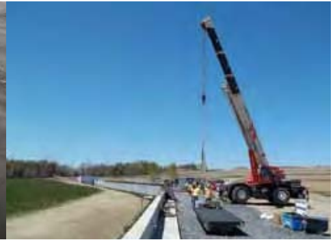
ARCHITECTURAL PRECAST CONCRETE WALL SECTIONS ARE BEING PLACED WITH A CRANE. Photo by Bryan Ciccocioppo, USACE
