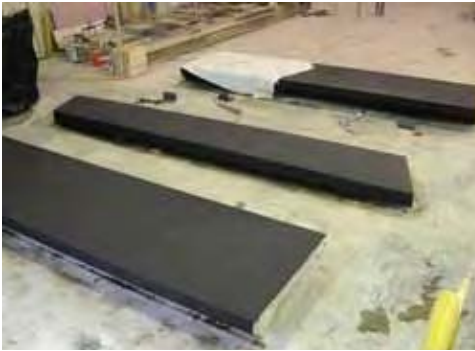
PRECAST CONCRETE WALL SECTIONS ARE SHOWN IN THE ROYAL STONE PLANT. Photo by Bruce Felix, Arrow Kinsley Joint Ventures
