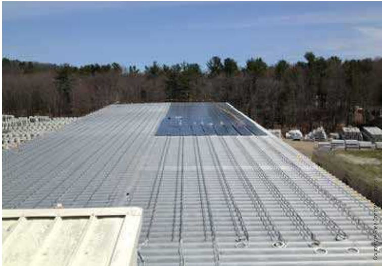
Solar panels were installed on Shea Concrete's Amesbury facility in 2013.
