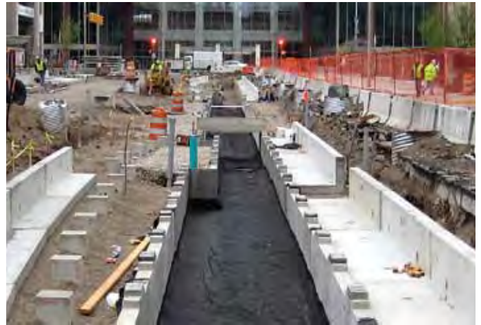
NORWALK CONCRETE INDUSTRIES – STORMWATER RECYCLING SLUICEWAY FOR PEDESTRIAN PROMENADE
