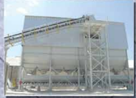
Weigh Belt Plant
