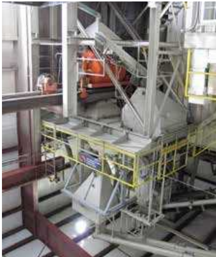
PLANT MODERNIZATION AT SHEA CONCRETE PRODUCTS, AMESBURY, MASS.
