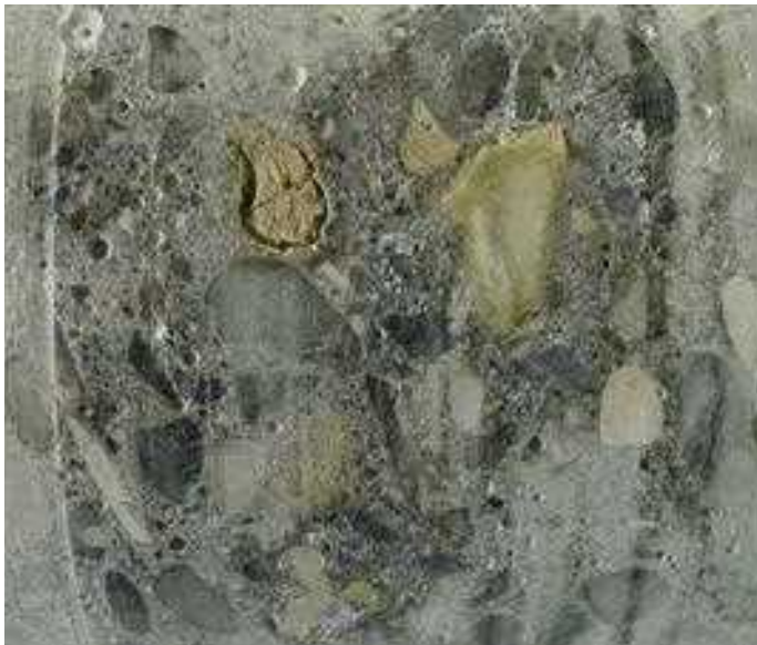
FIGURE 2. SEVERELY DEGRADED “SWEATY” ASR-REACTIVE AGGREGATE PARTICLES SHOWN ON THE EXPOSED SURFACE OF A CONCRETE CORE TAKEN FROM AN ASR-AFFECTED HARBOR WALL STRUCTURE. REACTIVE AGGREGATES WERE MAINLY COMPOSED OF POROUS CHERT. THE CEMENT PASTE SURROUNDING THESE REACTED AGGREGATE PARTICLES OFTEN APPEARS TO BE STAINED WITH ASR GEL, WHICH ALSO APPEARS AS A WHITE POWDER WHEN FULLY DRIED. Photo by Dr. Ted Sibbick, W. R. Grace & Co., www.grace.com
