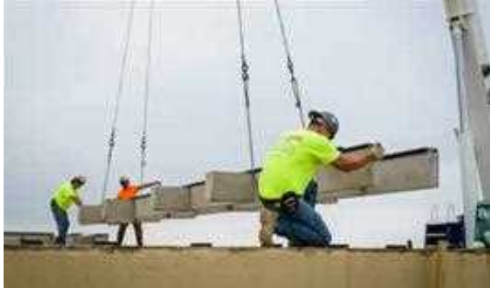
AFTER HURRICANE SANDY, PORTIONS OF THE BOARDWALK IN LONG BEACH, N.Y., WERE REBUILT WITH DURABLE PRECAST CONCRETE. Photo courtesy of US Concrete Precast Group
