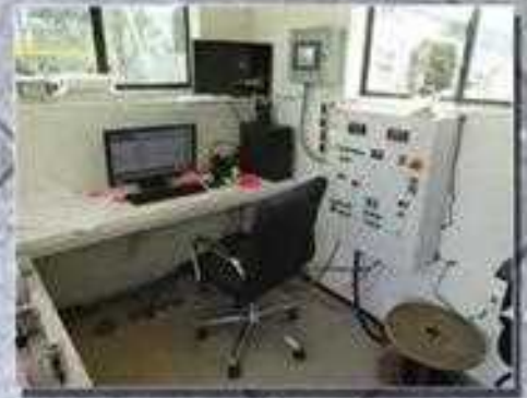
MPAQ Batching Automation
