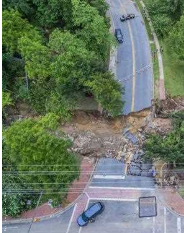
Flooding caused a large portion of Ellicott Mills roadway to wash away after an aluminum culvert installed beneath it failed.
