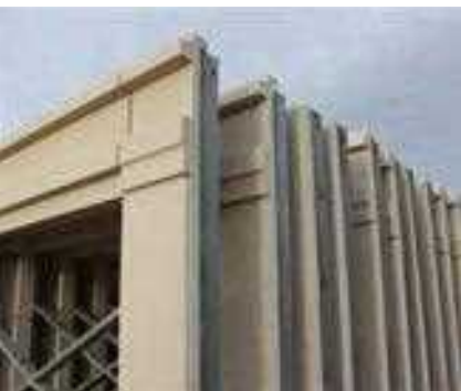
The goal for the Cliffside Park Towne Center project was to create the feel of a classic limestone building with a modern twist.
