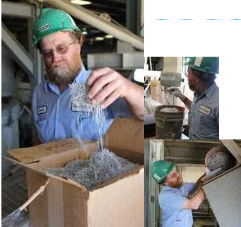
STEEL FIBERS ARE WEIGHED TO THE CORRECT PROPORTIONS THEN ADDED TO THE SCC MIX TO REDUCE THE AMOUNT OF REBAR REQUIRED IN THE FORMS. IN THE CASE OF THEIR STORM SHELTERS, LEE'S PRECAST USES THE STEEL FIBERS WITH NO REBAR AT ALL. Photos by Ron Hyink
