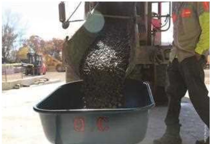
Collecting a representative composite sample is the first step in properly performing fresh concrete tests and fabricating compressive strength specimens.
