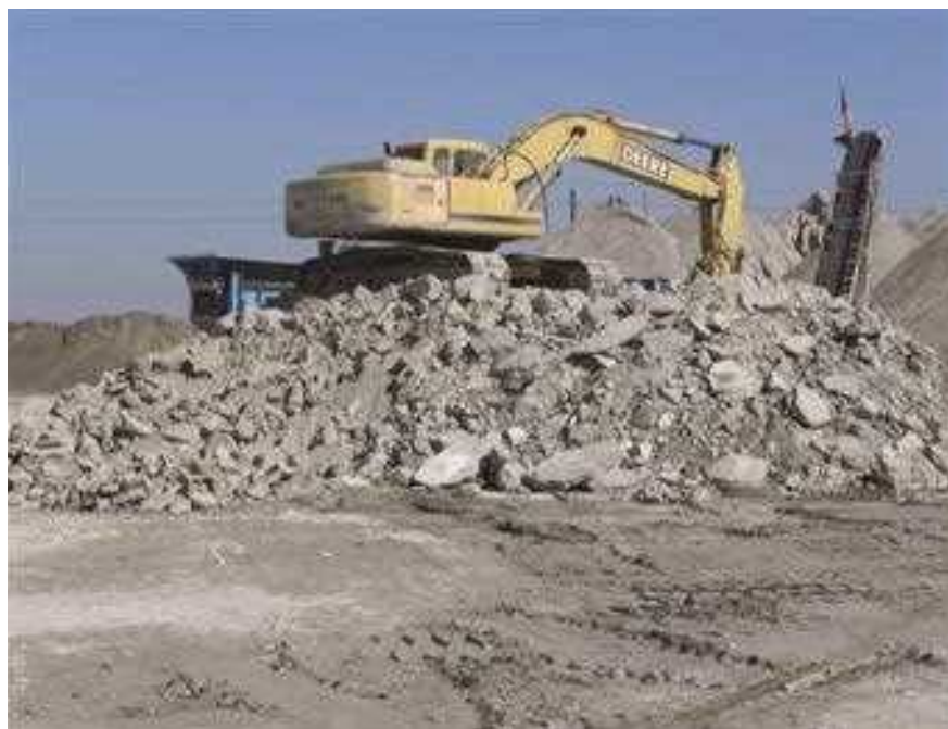
MATERIAL RECYCLING CENTER
