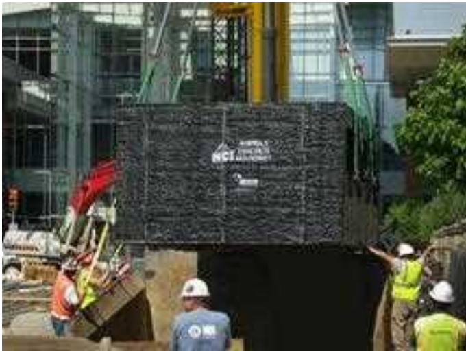
A UTILITY VAULT WITH A WATERPROOF COATING IS LOWERED INTO PLACE ON GEORGIA STREET IN DOWNTOWN INDIANAPOLIS.
