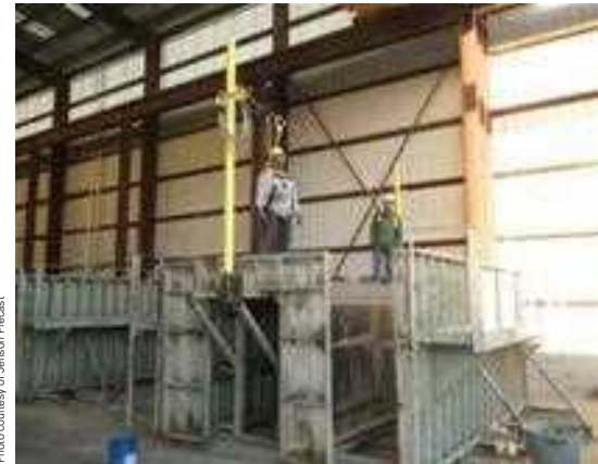
JENSEN PRECAST WORKERS WEAR FALL PROTECTION GEAR WHILE STANDING ON TOP OF PRECAST CONCRETE FORMS.
