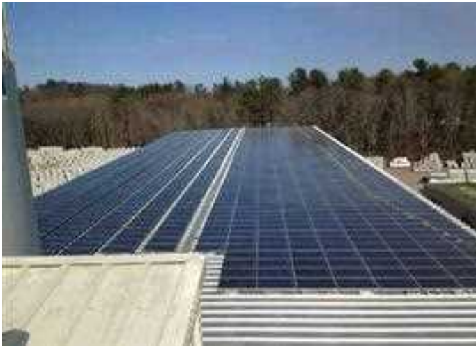
SOLAR PANELS AT SHEA CONCRETE PRODUCTS
