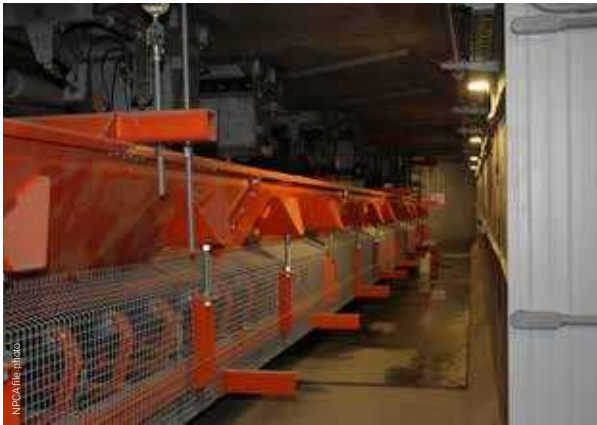
A precast concrete box culvert houses the company's underground aggregate weigh hopper.
