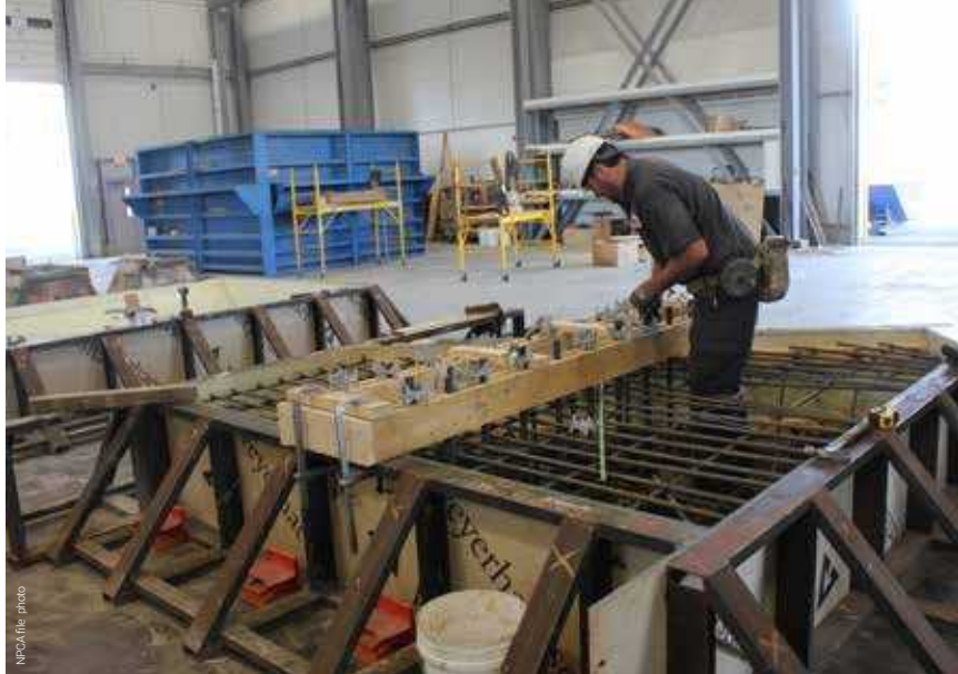
Camp Precast Concrete Products tackled more projects for the Vermont Agency of Transportation and the New York State DOT in 2017 than in past years.
