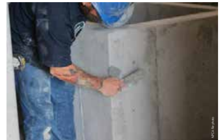
For buried concrete products structural and durability aspects of repair methods are the primary focus and not typically aesthetic concerns.
