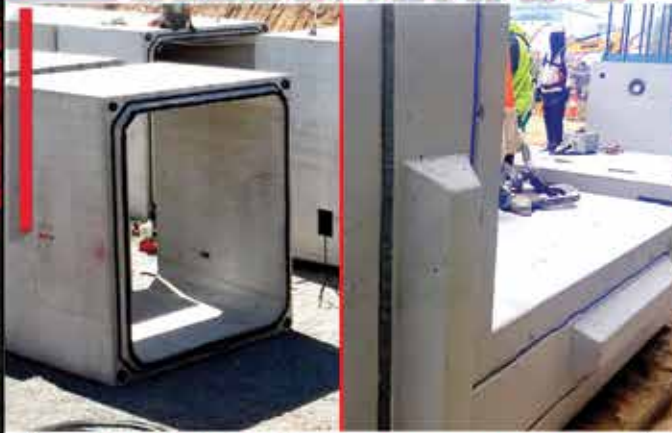
1 MILLION GALLON WATERTIGHT STORMWATER DETENTION SYSTEM
