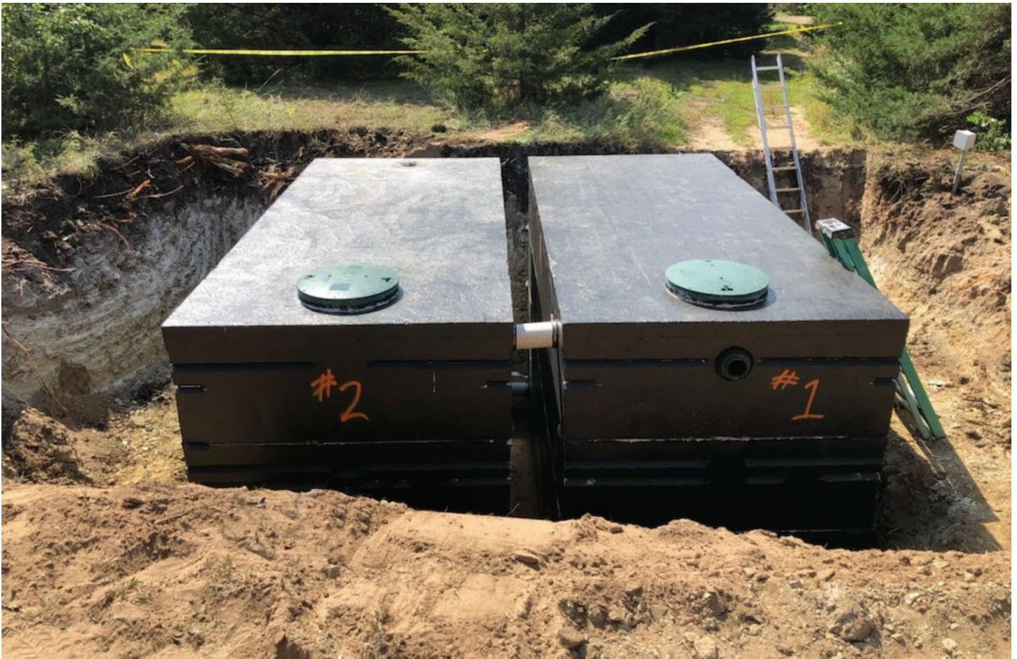
Figure 2: Example of close proximity equalization tanks with pipe connection
