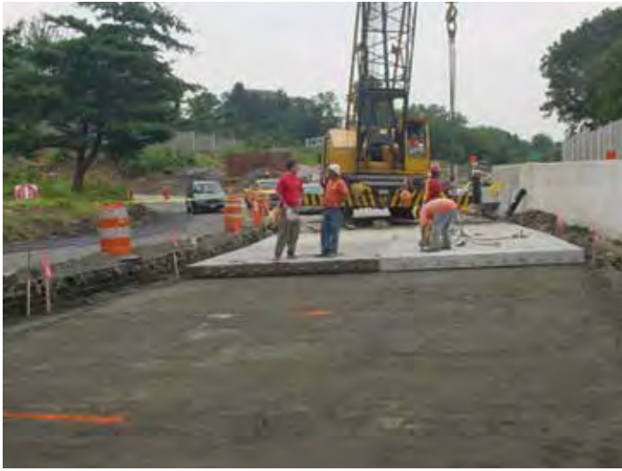
Figure 8-15. Panel points, identified with red paint, being used on a PCP project.
