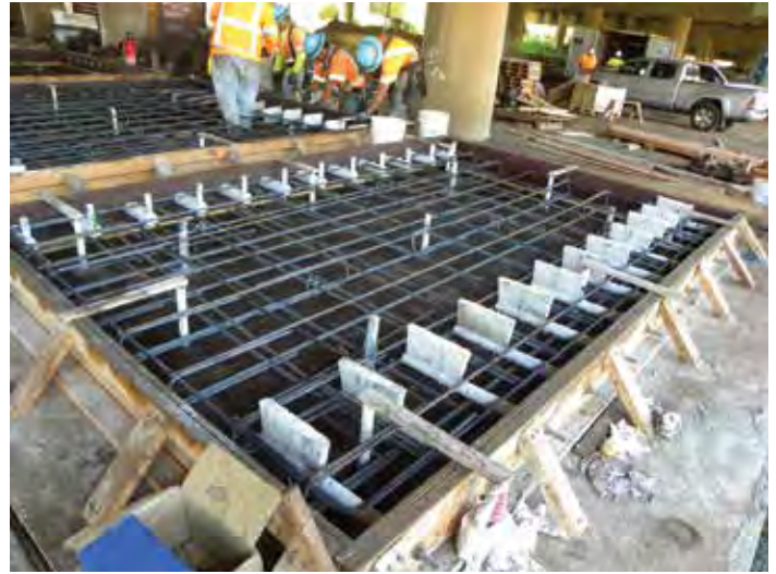
Figure 7-5. Plywood forms used at a contractor’s on-site “precast yard” under an overpass.
