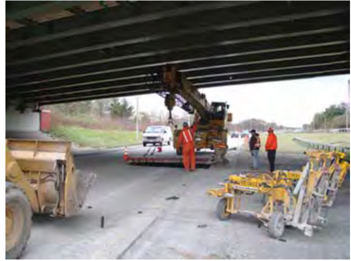
Figure 2-5. Example use of a crane placing PCP panels beneath an overpass. Traffic is maintained on the lane to the right of the excavator.
