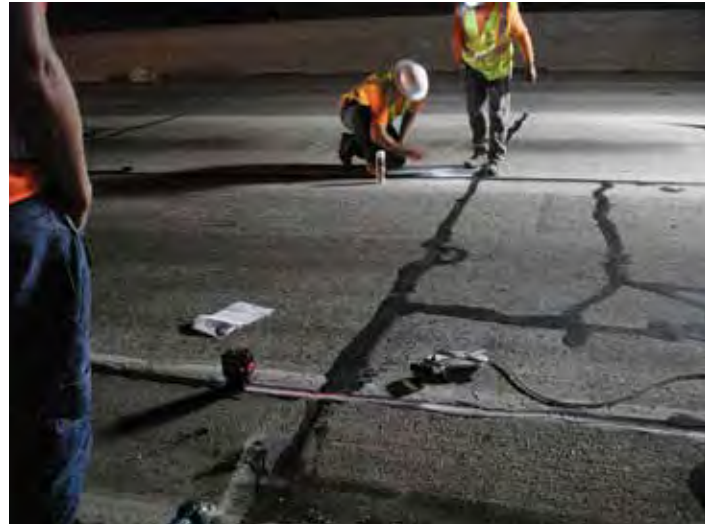
Figure 8-10. Workers using a right-angle laser tool to accurately mark a perpendicular transverse saw cut for a straight roadway.
