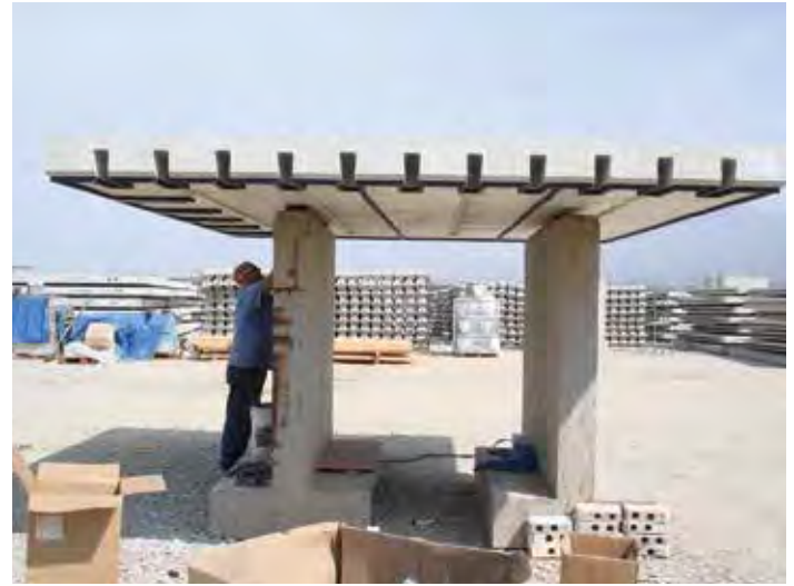
Figure 7-27. Applying foam gaskets to bottom of Super-Slab panels that have been placed on high stands.
