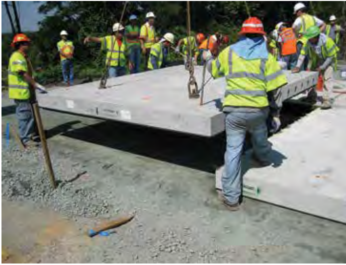
Figure 10-1. State DOT engineers witness the installation of a precast panel at a system trial installation.
