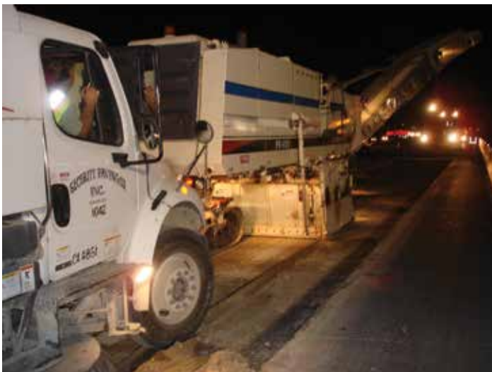
Figure 8-33. CTB removal with a large-scale milling machine, followed by a conventional "street sweeper" broom truck to ensure all milled material is removed.
