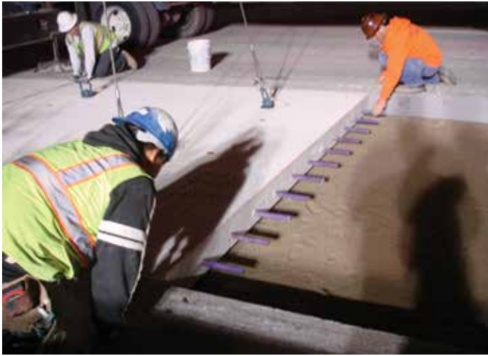
Figure 9-52. A PCP panel being placed to a leading end line stretched between two leading end marks.
