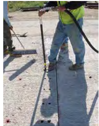
Figure 9-27. Injection of structural grout in dowel grout ports. Momentary pressure – to ensure the bottom slot is completely filled – is developed when an installer places a foot over the front port while dowel grout is pumped into the back port.
