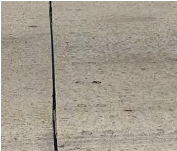
Figure 12-10. Grout in some dowel grout ports may have de-bonded here, potentially allowing water to penetrate to the dowel bar level.
