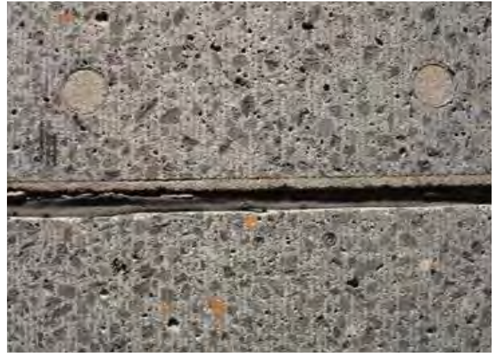
Figure 11-34. The sealant reservoir in this over-width joint was incorrectly cut with a 1/2-inch-wide blade. The remaining grout has already de-bonded from the existing pavement and is ready to fall out of the joint.
