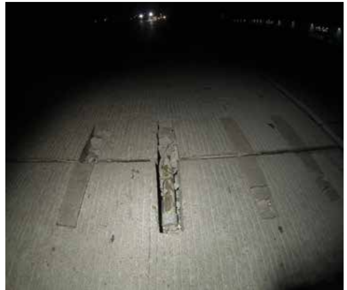
Figure 12-4. Bond failure between the grout encasing the dowel and the vertical sides of the slot.
