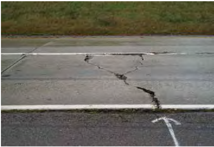
Figure 2-8. Deteriorating transverse crack on pavement.
