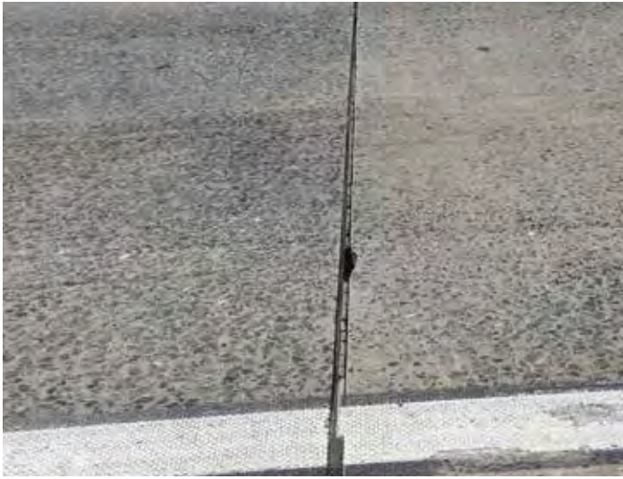
Figure 12-8. Joint-filling grout between the silicone seal on the left and the panel on the right has de-bonded from the panel, creating a maintenance problem in this variable-width joint.
