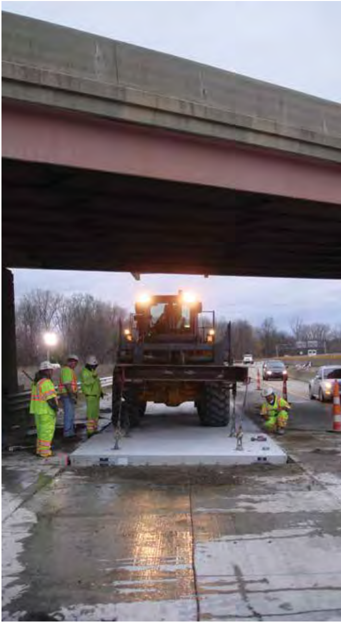
Figure 5-6. Example of a one-lane work area provided to replace the same lane.
