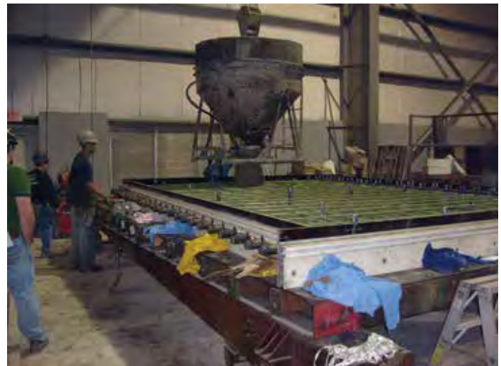
Figure 7-19. Use of a conventional concrete bucket to place panel concrete in a “high” form.
