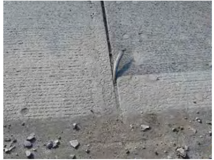
Figure 12-9. The bond between the silicone seal and concrete failed after approximately five years of service in this constant-width joint. Joint cleanliness problems during installation are suspected.
