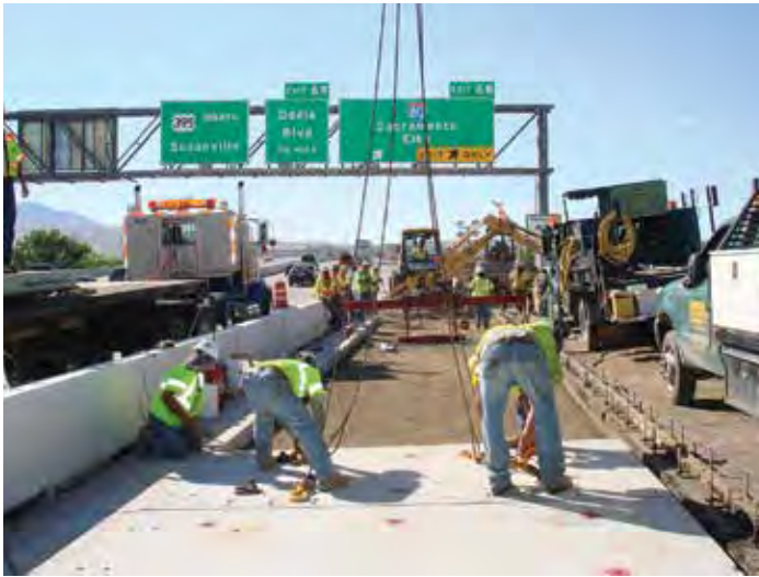
Figure 8-4. The work area allowed on this three-lane interstate was restricted to one lane, a small portion of the adjacent lane and the shoulder on the right.
