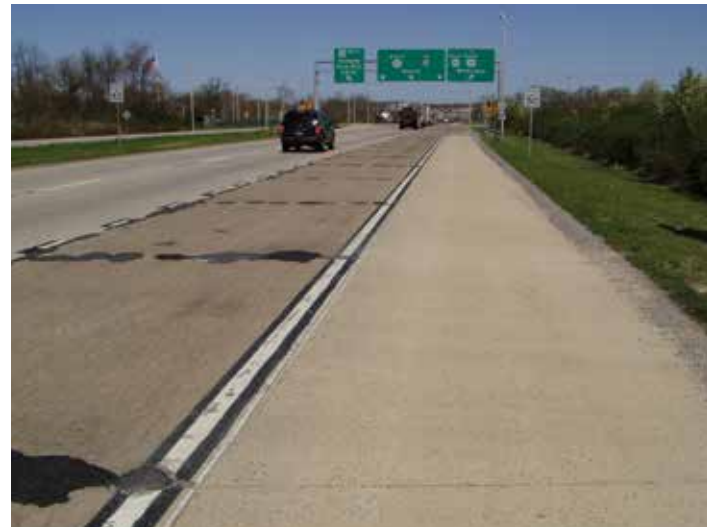
Figure 2-9. Joint failure on concrete pavement.
