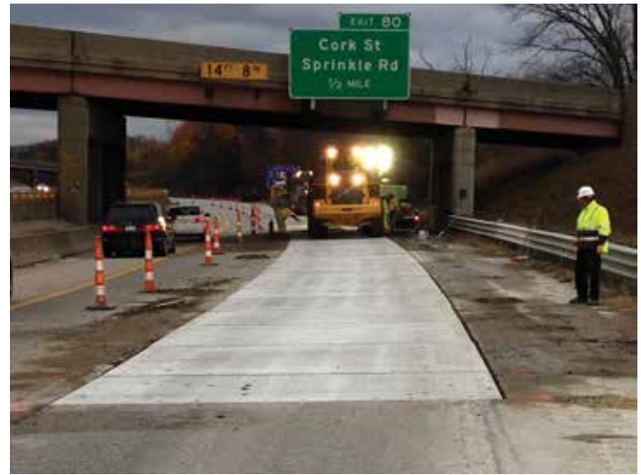
Figure 8-5. Traffic being diverted to the left shoulder, leaving a partial lane, a full lane and the shoulder on the right as a safe working area.
