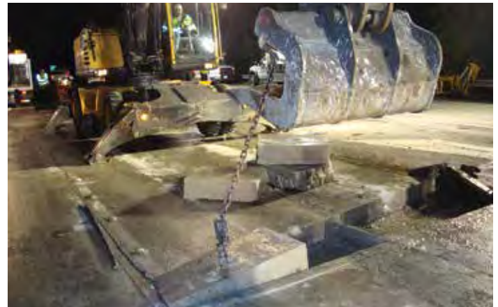
Figure 8-25. Excavator removal using a slab-crab bucket, showing little disturbance of the underlying subbase.
