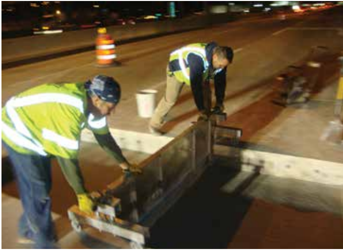
Figure 9-1. Screeding device using adjacent existing pavement as the frame of grade reference.
