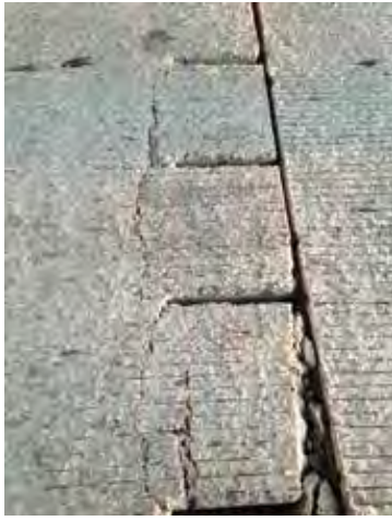
Figure 11-15. This photo shows a cast-slide panel that shattered around the dowels before the slots were grouted.
