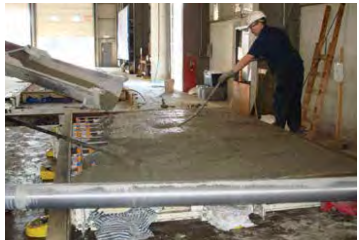
Figure 7-20. Concrete placement directly from a ready-mix truck (form is low enough to permit direct placement from the truck).
