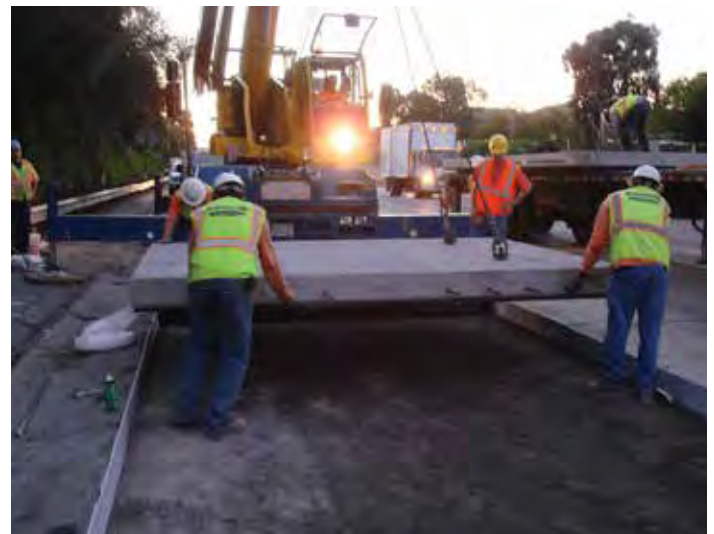
Figure 10-16. An ideally sized panel placement crew of five, with one man in each corner and one man on the truck.
