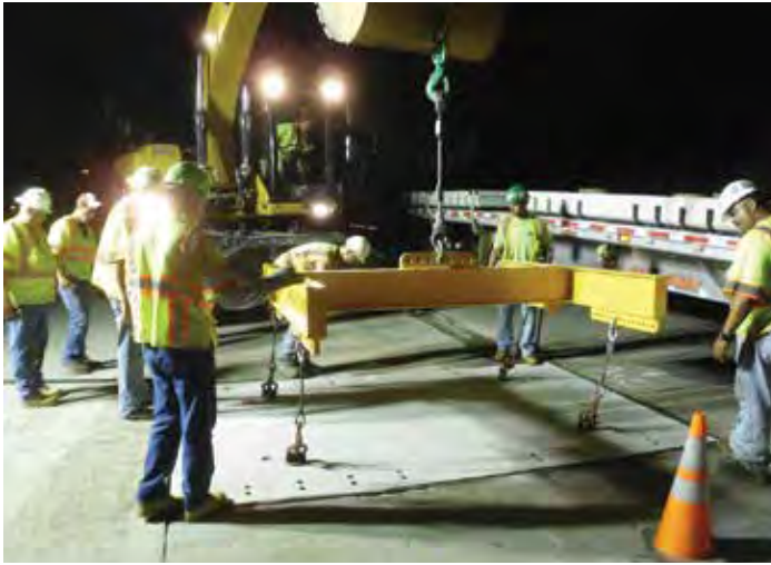
Figure 9-45. A rubber-tired excavator placing a 12-foot-wide-by-10-foot-long panel that was “picked” from the truck positioned alongside.
