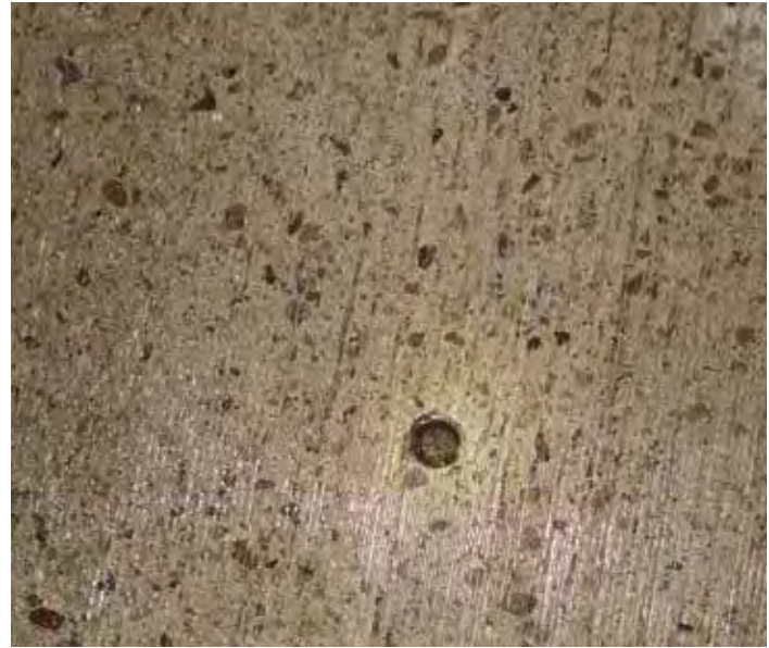
Figure 12-11. This bedding grout port was not properly filled during initial panel installation.
