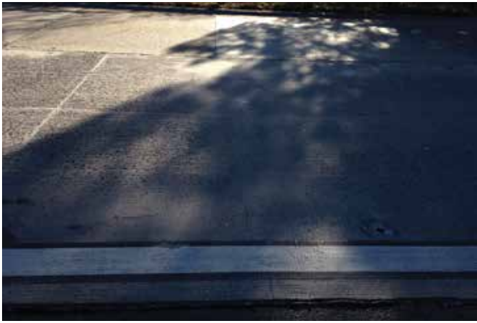
Figure 11-6. A transverse crack in the foreground lane lines up approximately with a joint at a cast-in-place concrete patch in the adjacent lane.
