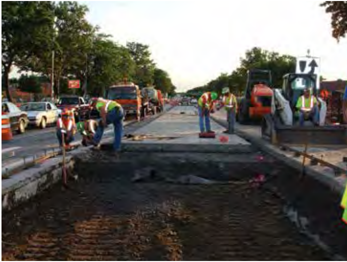
Figure 2-12. Undercutting foundation prior to placing PCP panels on Route 7 near Rotterdam, N.Y.
