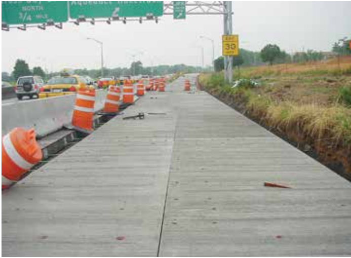
Figure 4-4. Wide precast concrete ramp pavement in Long Island, N.Y., with a longitudinal joint in the center of the lane.
