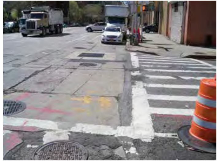
Figure 2-17. Urban intersection requiring repair with numerous utility access points.
