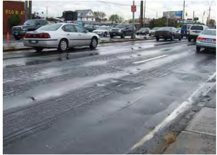
Figure 3-17. Heavily rutted asphalt pavement on Rockaway Boulevard in Queens, N.Y.
