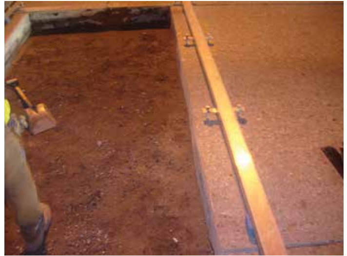
Figure 8-18. An undulating vertical saw cut made with a blade that was likely too flexible for the pavement.
