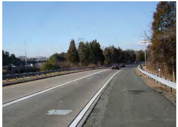
Figure 3-11. The right-hand lane of a high-speed exit ramp in Fairfax, Va., that was replaced during overnight full ramp closures.
