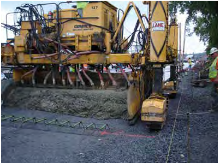
Figure 1-3. String line controlled slip-form paver approaching dowel basket (note vibrators for consolidation).
