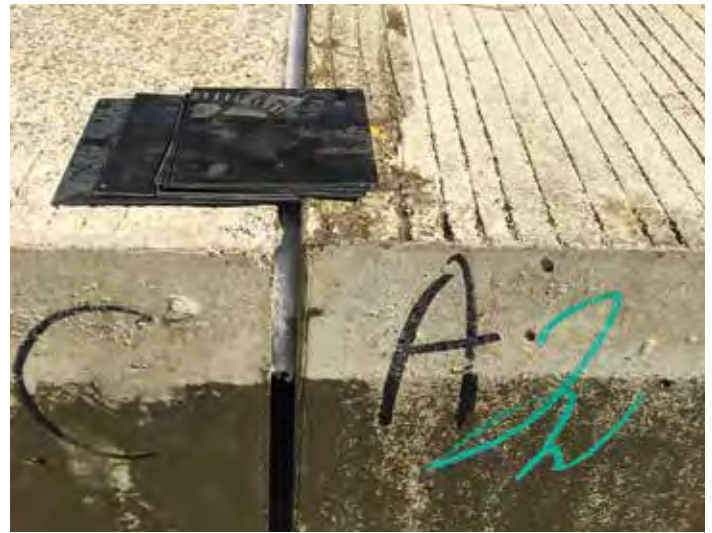
Figure 10-9. Two shims left behind indicate an actual vertical differential of 1/8 inch between the two panels.
