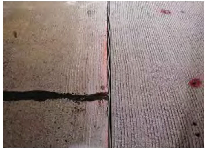
Figure 11-30. The isolation foam in this longitudinal joint does not completely fill the joint.
