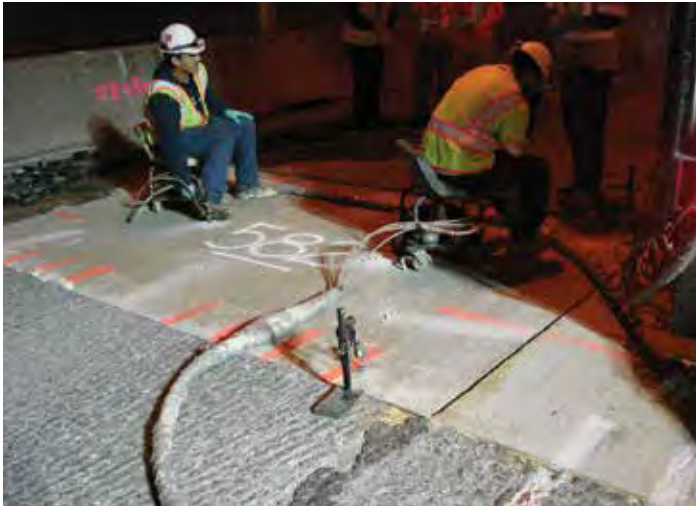
Figure 9-11. Two workers, each equipped with a urethane injector tip, installing foam to the underside of the panels through foam ports.
