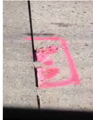
Figure 11-4. Photo showing failure of backfill material in top slots around the dowels and failure of the concrete between the slots.
