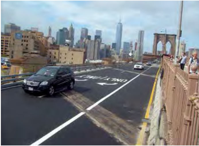
Figure 3-19. Only the header portions of the skewed precast approach slab panels used on this Brooklyn Bridge project in New York City are visible in this photo. All other precast panel exposures were overlaid with asphalt to provide a smoother riding surface.
