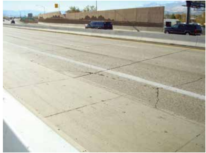
Figure 2-13. Precast panels placed next to cracked pavement on Interstate 395 near Reno, Nev.
