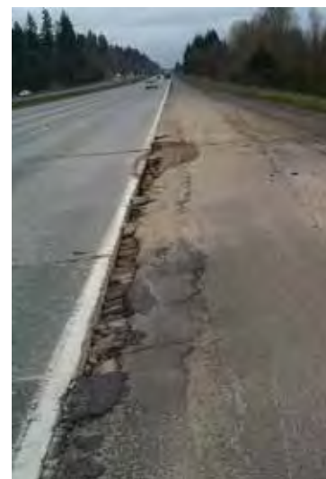
Figure 2-11: Joint and crack faulting with severe pumping, indicating drainage and erosion problems.
