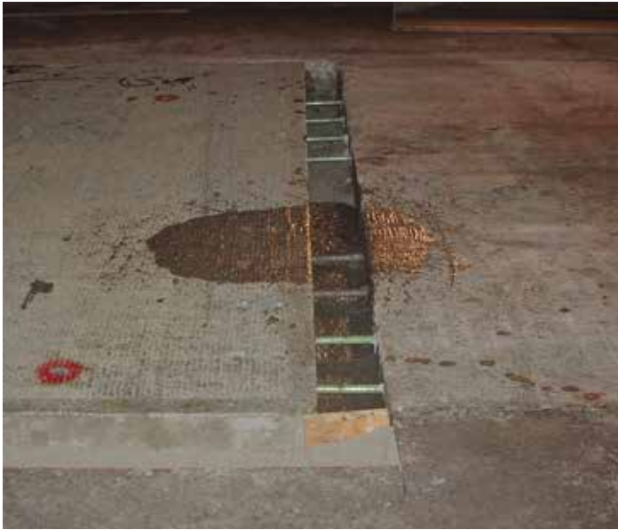
Figure 12-5. This excessively wide transverse joint resulted from cutting the existing pavement (on the right of the joint) at the incorrect location. The dark material at the center of the joint is backfill grout that spilled onto the adjacent slabs during installation.
