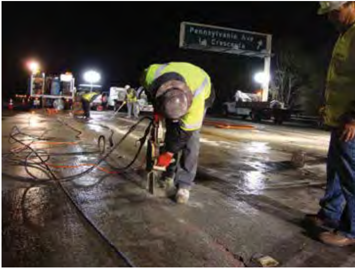
Figure 8-20. A concrete chainsaw equipped with diamond teeth is used to finish a full-depth saw cut without overcutting into the adjacent panel.
