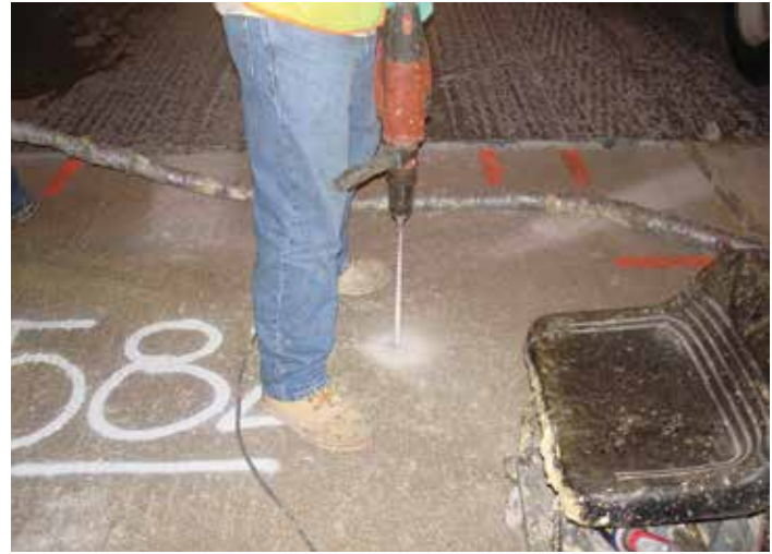
Figure 9-12. A worker drills a new foam port in a part of the panel that needs extra force to provide vertical uplift.
