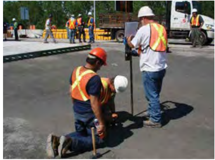
Figure 8-16. Survey crew using a robotically controlled total station to lay out panel points on a total replacement project.
