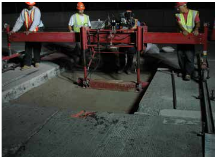
Figure 11-1. The relatively thin spall in the existing pavement seen along the longitudinal joint in the lower-right corner was caused by improper removal techniques.
