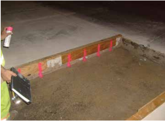
Figure 9-25. The template seen here consists of pre-drilled plywood supported by an attached 2-inch-by-4-inch horizontal member.
