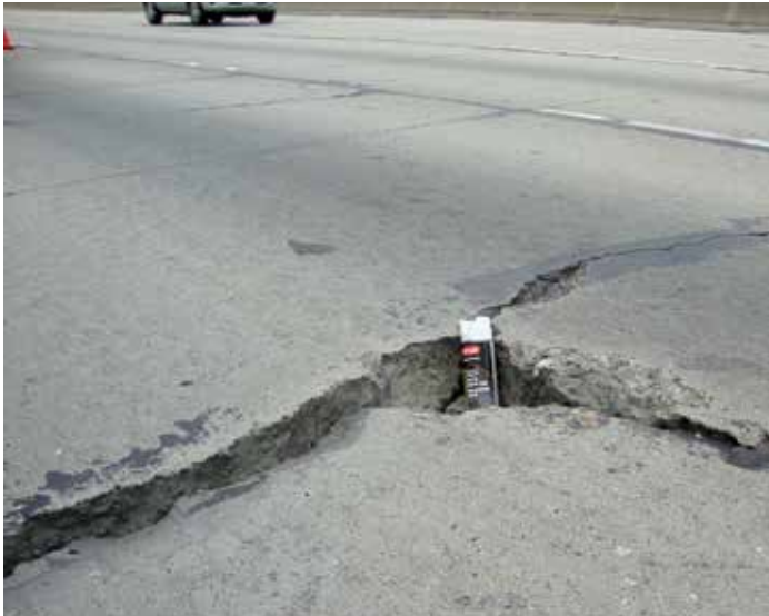
Figure 1-1. Photo of deteriorated concrete pavement.
