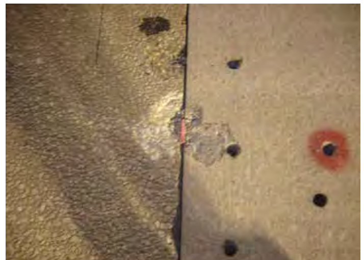
Figure 11-2. Transverse joint spalls in both the existing pavement and the new precast panel in this photo resulted from the red shim pad – placed to keep adjacent panels from hitting each other – being placed too close to the surface.
