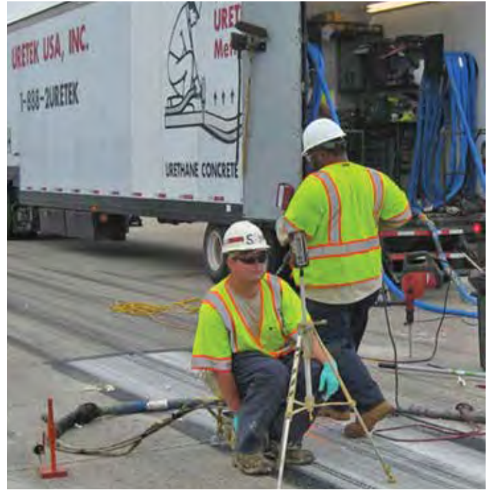
Figure 9-20. A fully equipped urethane injection support truck is seen in the background.
