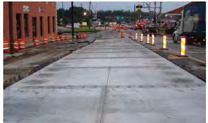
Figure 11-25. Severe cross-slope and vertical profile grade changes at the far end of new panels.
