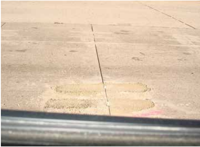
Figure 11-5. The original dowels in the top slots seen in the foreground were sawed out and replaced with new, full-length dowels and the slot was backfilled with polyester concrete.
