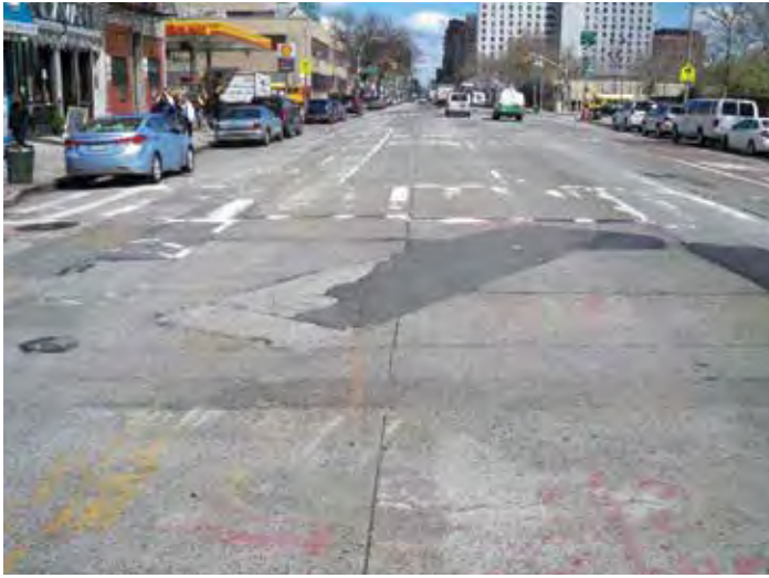
Figure 13-10. An example of city street pavement with many utility cuts (First Avenue, New York City).
