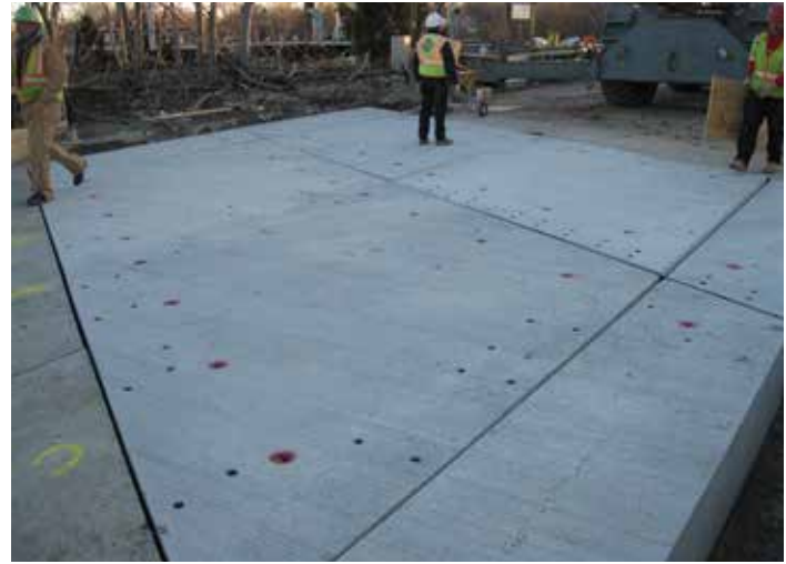
Figure 3-23. New precast concrete bridge approach panels at the Route 46 Bridge in Clifton, N.J.
