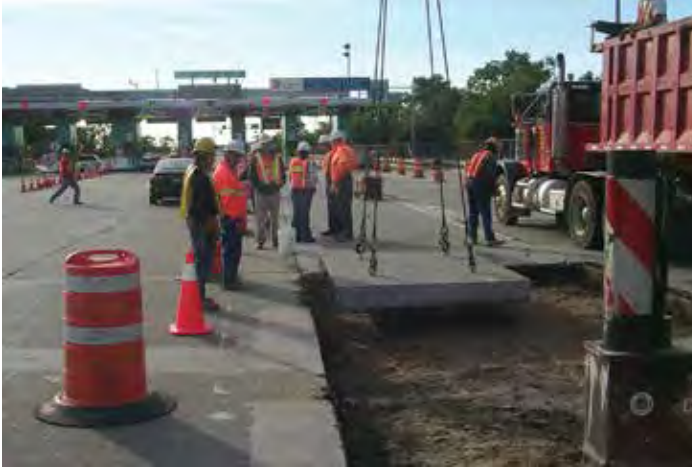
Figure 8-22. Slabs being removed using the lift-out method. Notice the spalls on the edge of the remaining pavement on the left caused by the lifting operation.
