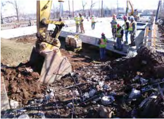
Figure 3-22. Replacement of bridge embankment material below approach slabs on the Route 46 Bridge in Clifton, N.J.
