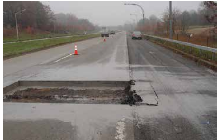
Figure 8-14. Failure to cut the asphalt shoulder prior to pavement removal resulted in serious shoulder damage on this project.
