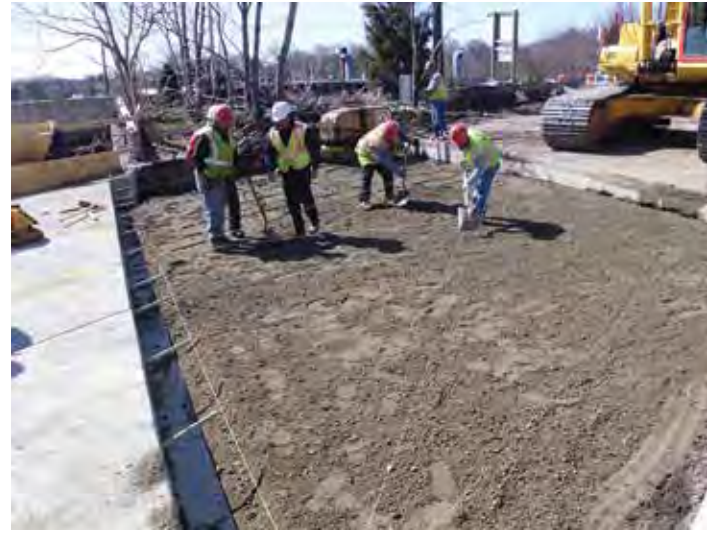
Figure 10-15. A grading crew using string lines (foreground) to check the rough grade of bedding material.
