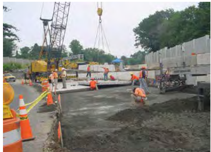
Figure 9-49 Because equal-length picking cables were used over a sloped surface, PCP panels on this project had to be placed numerous times to bring joint widths within specified tolerances.
