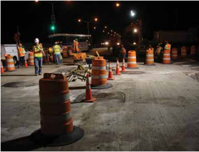
Figure 2-18. Numerous utility blockouts in precast panels temporarily filled with asphalt to maintain traffic.
