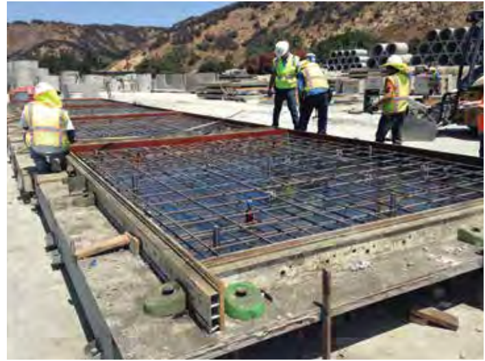
Figure 7-9. Aluminum extrusions (faced with special plywood) anchored with magnets in a long-line bed.
