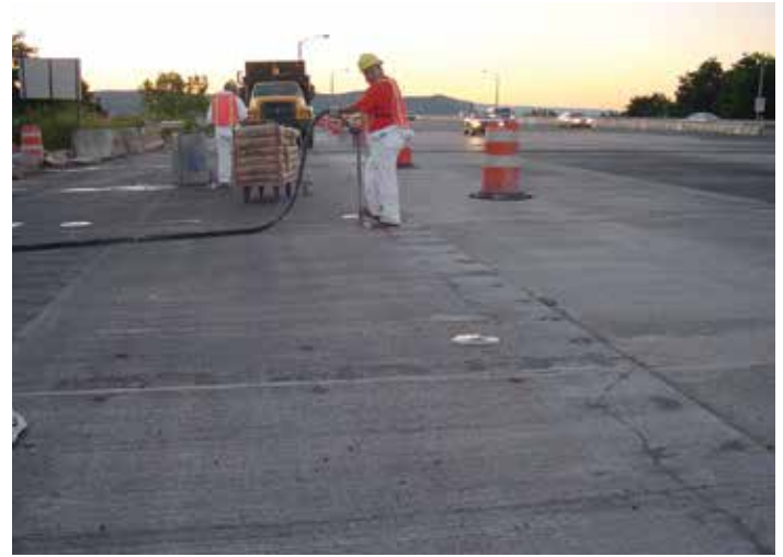
Figure 9-18. A worker pumping bedding grout into one end of a distribution channel until it comes out the other, a technique that verifies bedding grout has flowed under pressure for the entire length of the channel, indicating full distribution of grout under the panel.
