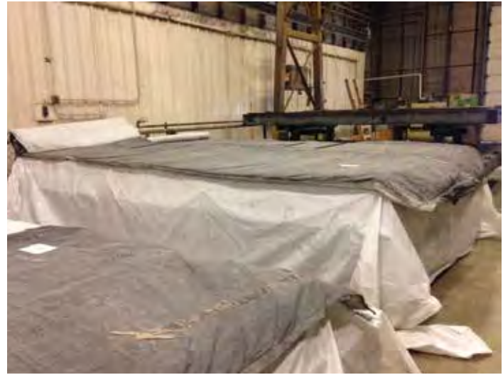
Figure 7-25. A newly casted panel covered with plastic and insulating blankets for initial curing.
