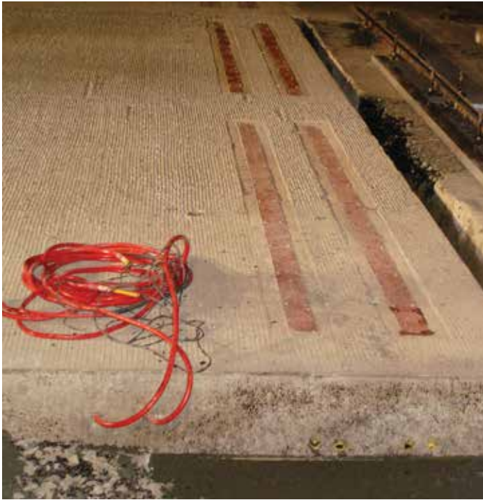
Figure 13-23. Construction photo showing night-time installation of an open-road-tolling precast panel at a New York State Thruway toll plaza in 2006.
