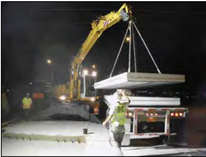
Figure 6-4. Rubber-tire excavator placing a 12-foot-wide-by-10-foot-long panel. The same equipment was also used to excavate and remove the existing pavement.
