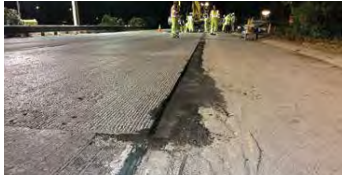
Figure 11-37. This new asphalt – placed directly against new precast panels – was barely wide enough to allow proper and uniform compaction.
