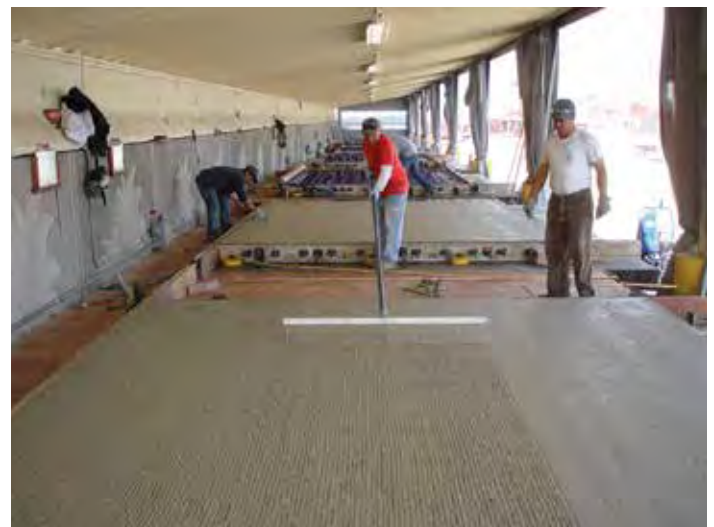
Figure 7-23. Commercially available rake being used to impart macrotexture on top of a previously applied burlap drag ("microtexture") finish.
