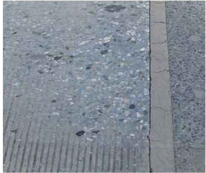
Figure 12-6. Hairline cracks in a 2-inch-wide grouted joint between two precast panels.
