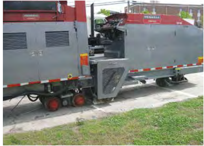
Figure 11-22. Typical diamond grinding profiler with grinding head near the center of the photo. The bogie wheels on the left control the cross-slope of the head while the dual in-line center wheels on the right establish the longitudinal profile of the grinding machine.
