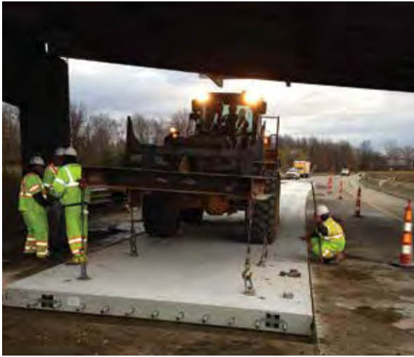
Figure 3-26. Placement of repair panels beneath an overpass on westbound Interstate 94 (Business Loop) near Kalamazoo, Mich.
