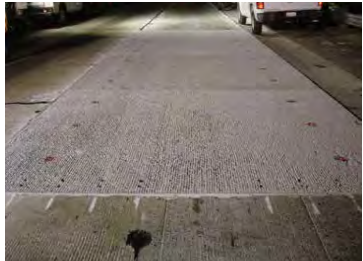
Figure 11-27. These panels, finished at the precast plant with a burlap drag-and-raked finish, did not require diamond grinding. Friction requirements were met during panel fabrication and smoothness requirements were met during panel placement.
