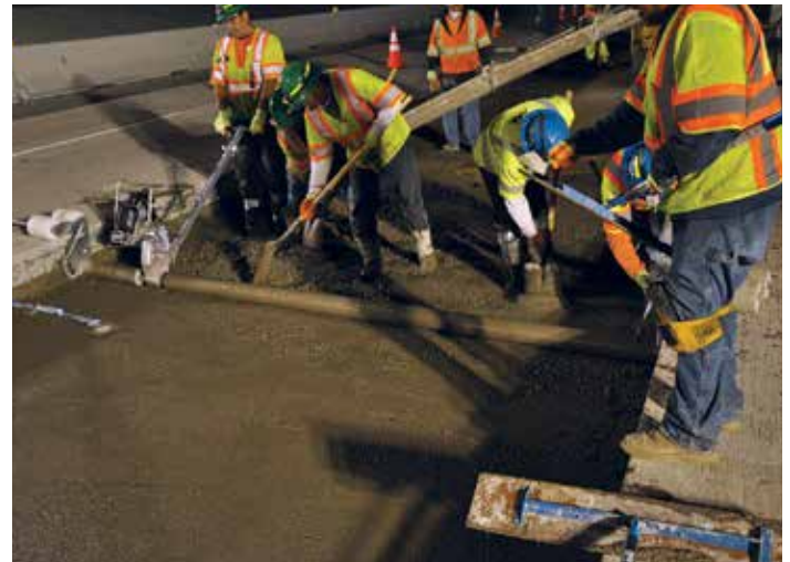
Figure 9-8. A "homemade" mechanized roller screed is used to screed new lean concrete base while masons hand-finish the new lean base on each side of the placement.
