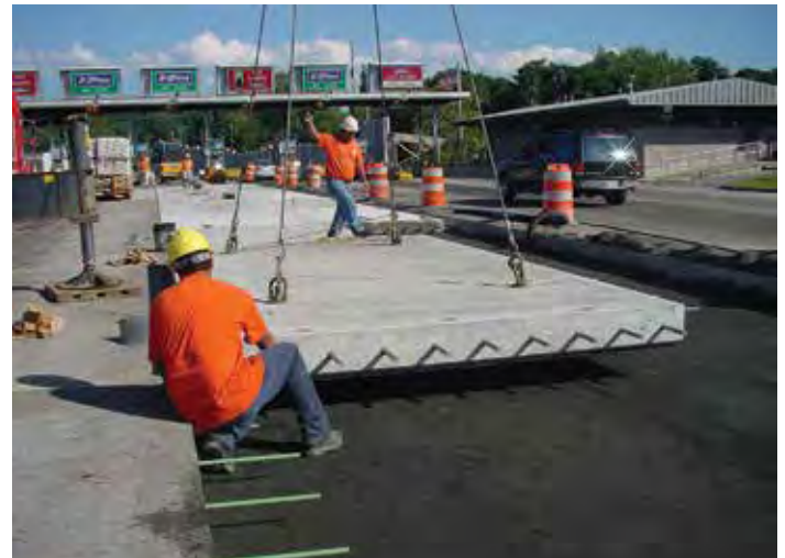
Figure 4-9. Placement of grade-supported precast panel for overnight use prior to installation of bedding grout at Tappan Zee Toll Plaza in New York.
