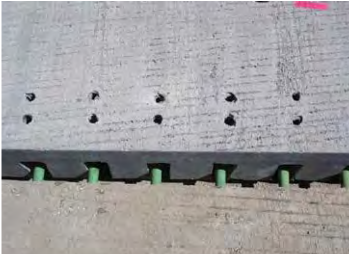
Figure 9-23. A precast bottom-slot (Super-Slab) panel being lowered over the dowels of a previously placed panel.
