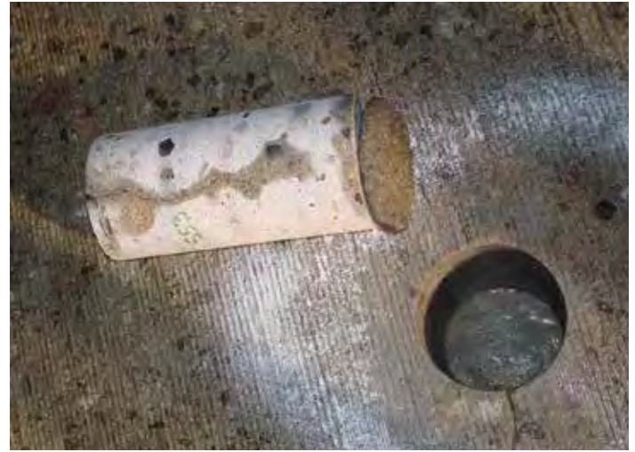
Figure 11-10. The crack in this core measured .06 inches wide at the top of the core and stopped at the bottom layer of reinforcing.
