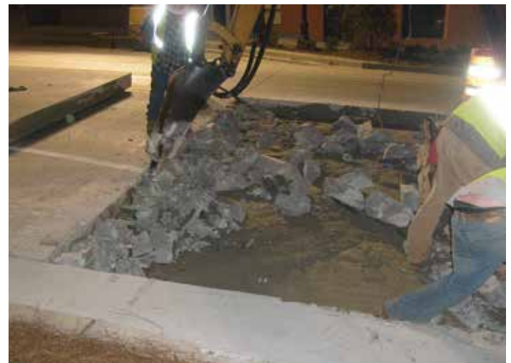
Figure 11-20. A small hoe ram removing concrete around dowels that are to remain in place.
