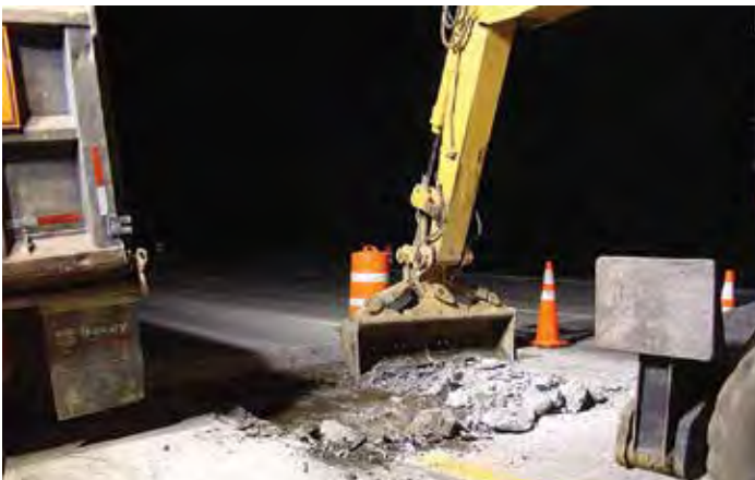
Figure 8-24. The shattered pavement seen here had to be removed with an excavator even though the lift-out method was specified.
