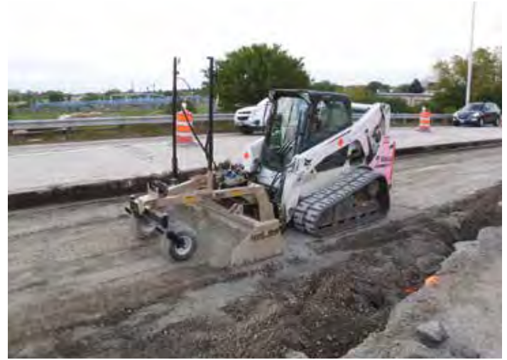
Figure 9-4. A laser-equipped skid-steer and grading box using a digital surface model for grade control.
