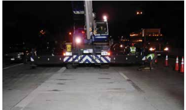
Figure 8-1. Men working approximately 8 feet away from live traffic, separated only by widely placed traffic cones.
