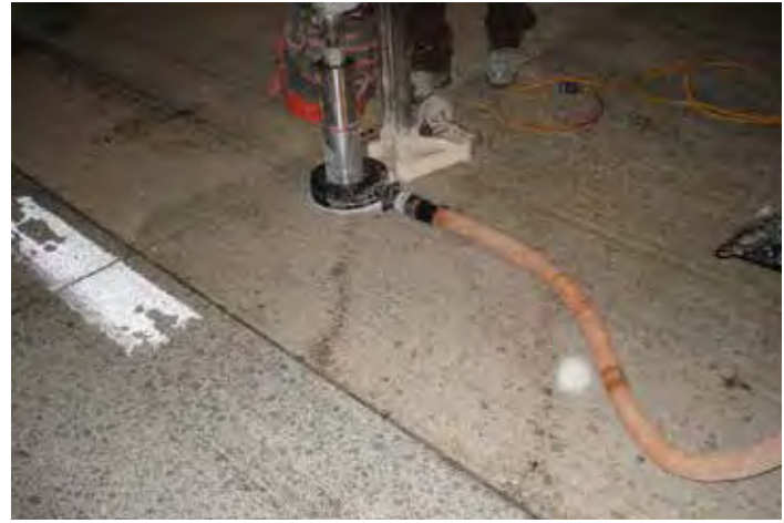
Figure 11-7. This diagonal crack – visible because it is wet – emanated from a bottom slot directly under the core drill. The crack was likely caused by inadequate corner support resulting from improper grading and/or installation of bedding grout.
