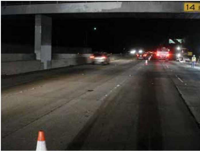
Figure 8-2. The work area on this five-lane California interstate project was three lanes wide, providing a safe, 12-foot-wide buffer zone.
