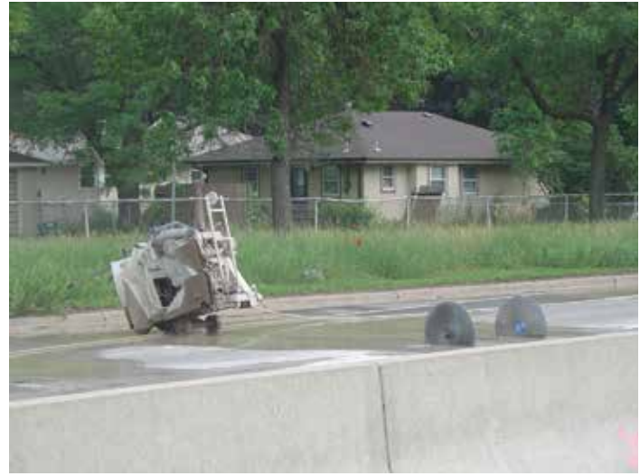
Figure 8-21. Saw blades bound up by slab expansion in hot weather.
