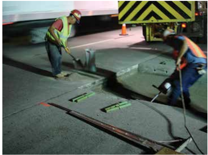
Figure 8-3. The narrow buffer zone in this two-lane working area required workers to exercise extreme caution.
