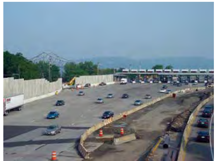
Figure 3-21. The expanded Tappan Zee Bridge toll plaza after precast panel installation was completed in 2002 (photo taken during off-peak hours to highlight the expanse of precast panels).
