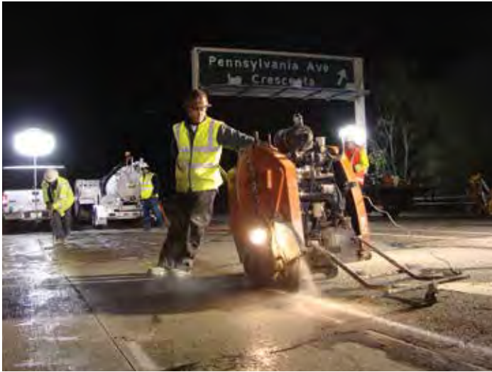
Figure 8-17. This sawing crew is equipped with adequately sized saws, proper lighting, a water supply and a slurry suction truck.
