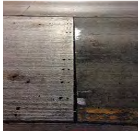
Figure 11-12. The transverse joint seen here varies in width from about 1/2 inch on the far end to approximately 2 inches on the near end because of incorrect saw cutting of the existing pavement.
