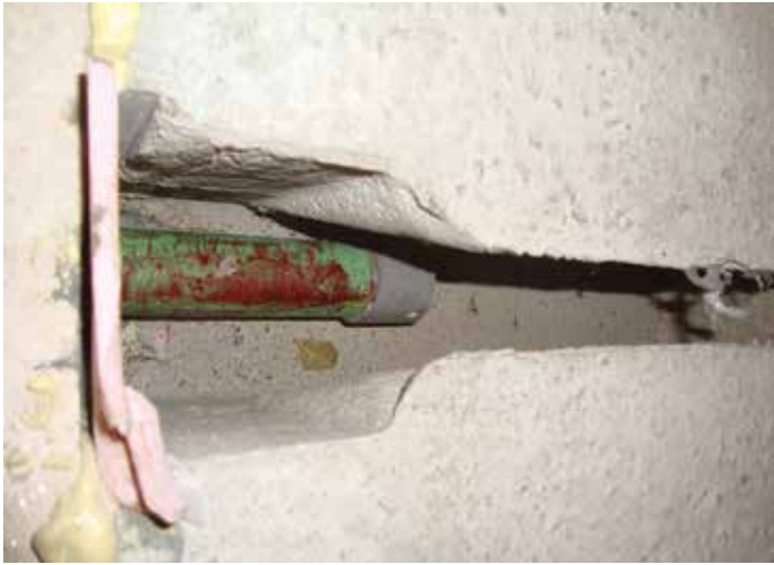
Figure 9-34. The hole drilled for the dowel in this photo was not closely aligned with the cast-in slot, making dowel installation difficult.
